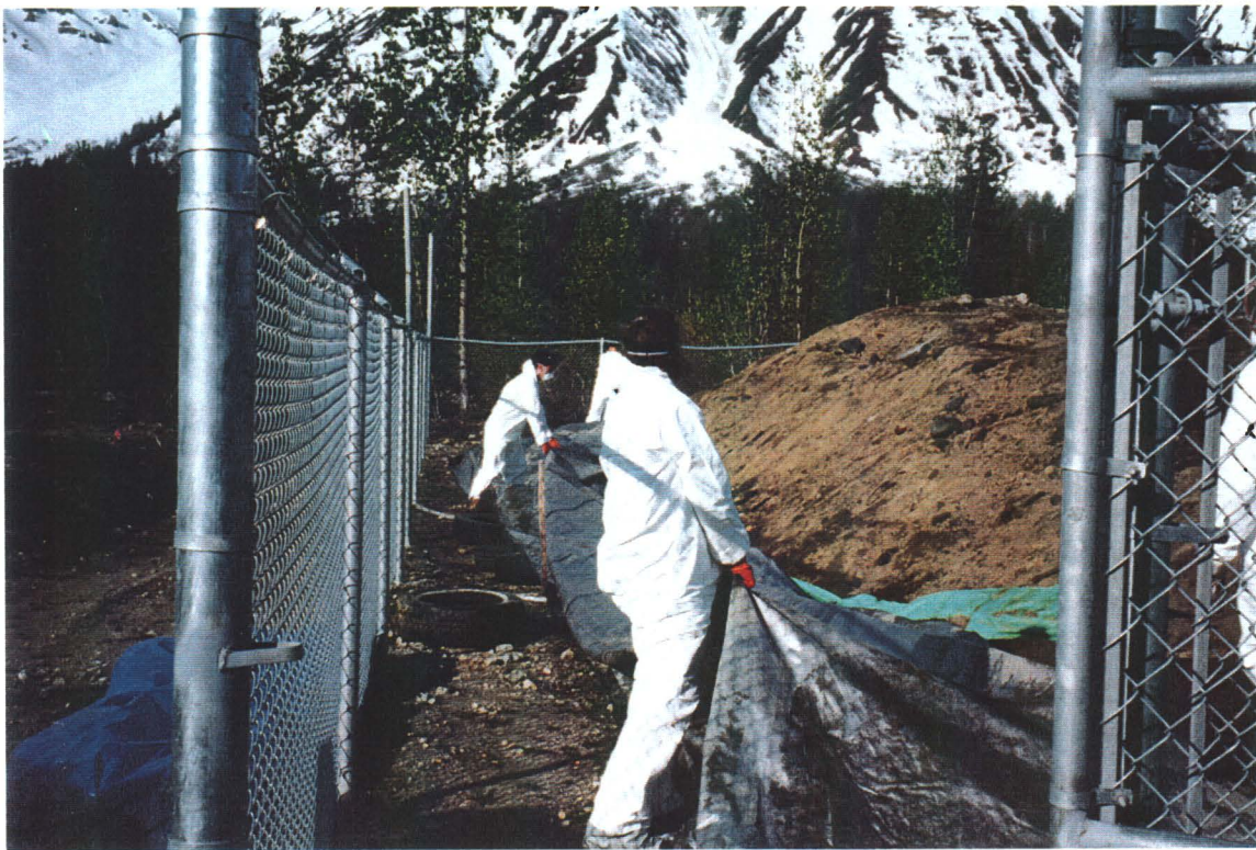
Photograph 2.2: Removing tarpaulin coverings from the DDT contaminated soil at the Temporary Storage Facility
