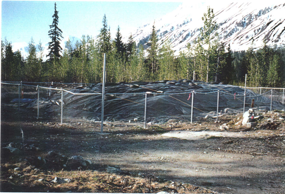
Photograph 2.1: Temporary Storage Facility showing fence and DDT contaminated soil with tarpaulin covering
