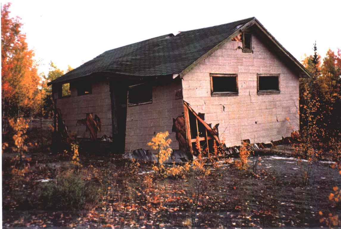
SITE 16 - Damaged building - interior paint sample obtained
