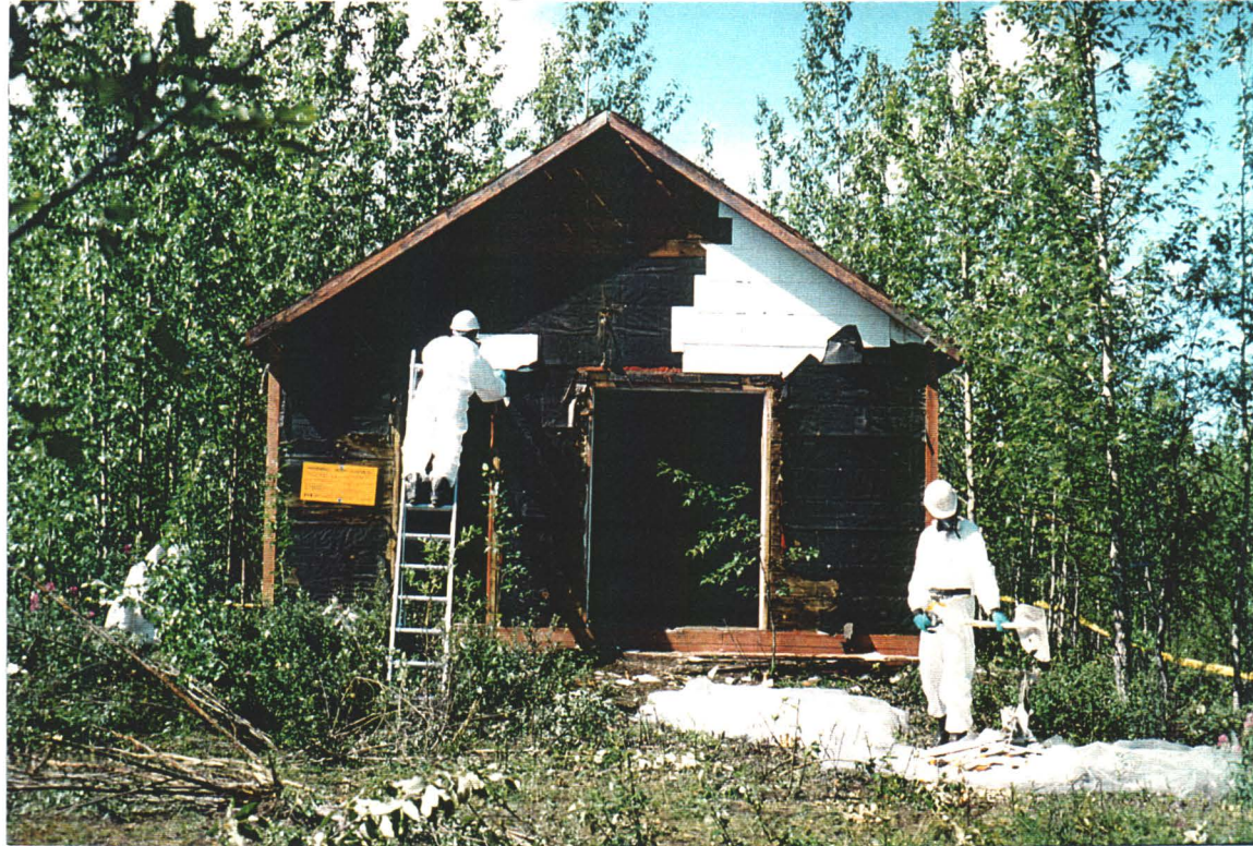
PHOTO 5: Firehall -Removal of asbestos containing roof tiles and exterior building shingles. Tiles and shingles were double wrapped in polypropylene.
