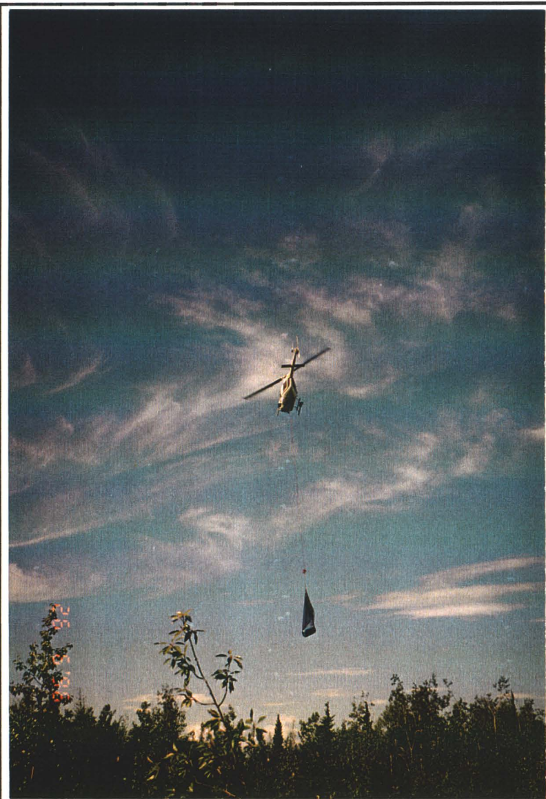
PHOTO 8: Beacon Site - Excavated soil, painted wood and metal debris were slung by helicopter to the temporary staging cells, where the the nets were unloaded.
