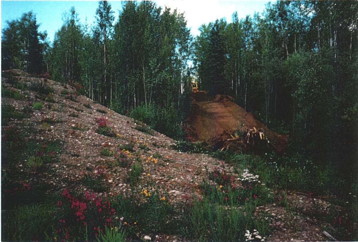
PHOTO 10: Landfill - Unpaved road constructed from road leading into landfill to the toe of the landfill. Photograph taken from toe of landfill.
