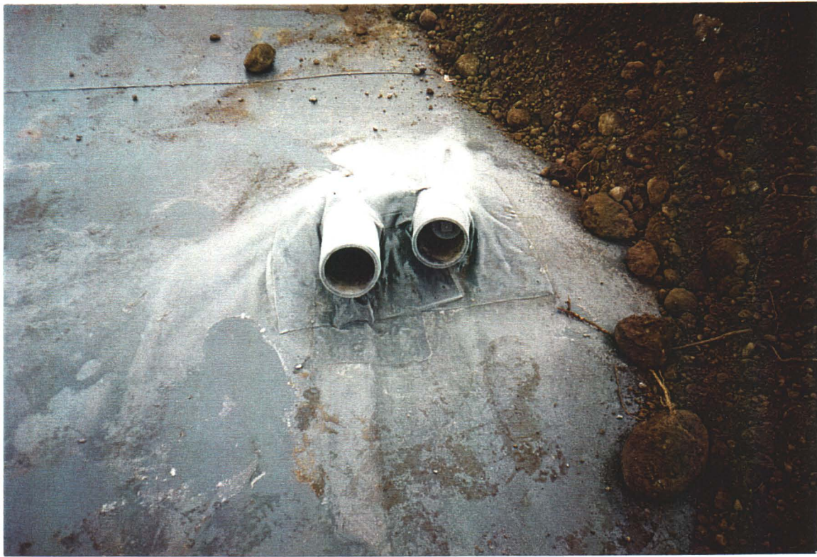
PHOTO 13: Containment Cell - Two monitoring wells in containment cell. Note: Liners were sealed around protruding pipes with custom fabricated boots.
