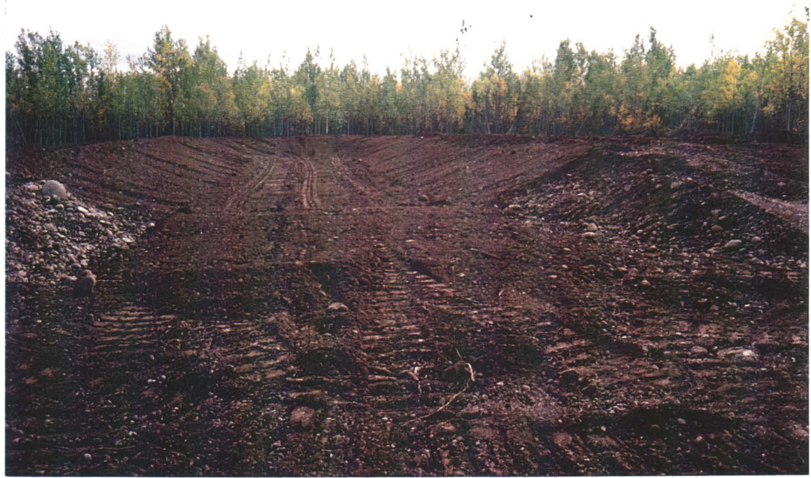
PHOTO 11: Containment Cell - Containment cell with compacted berms subsequent to grading. View looking east.
