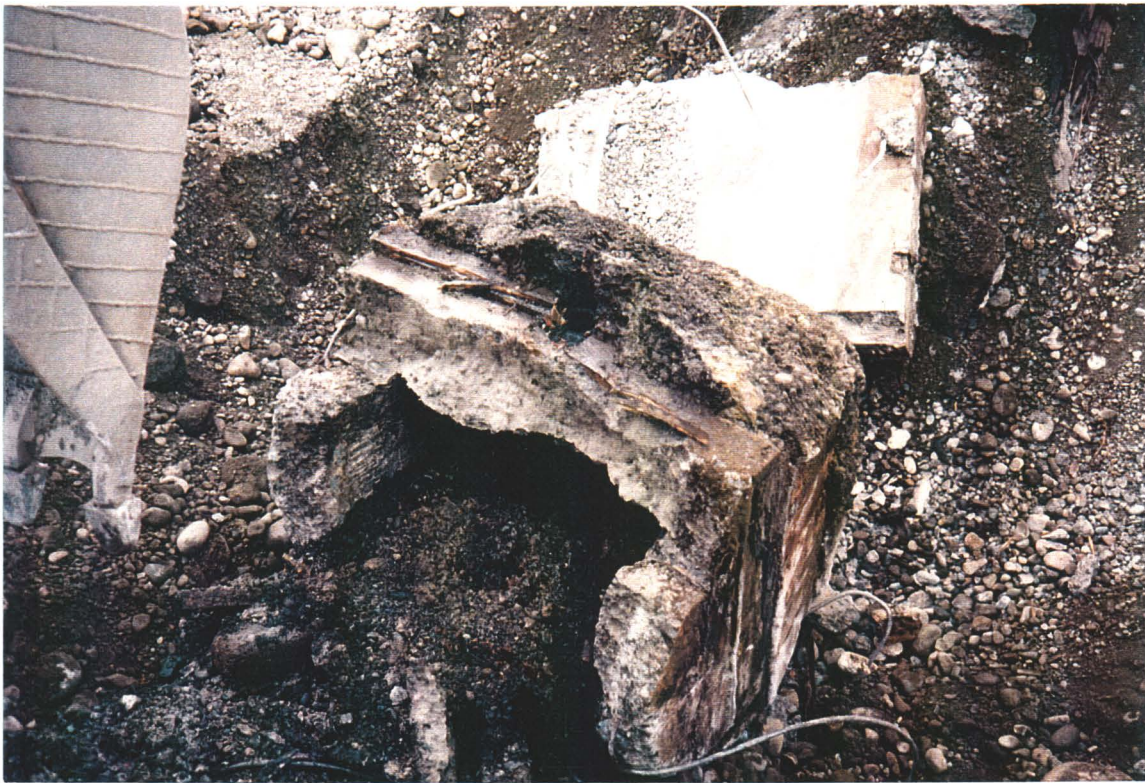
PHOTO 7: Garage - Concrete sump from garage pit. Note, black sludge in sump. NOTE: This sludge was removed and placed in secure barrels for disposal.
