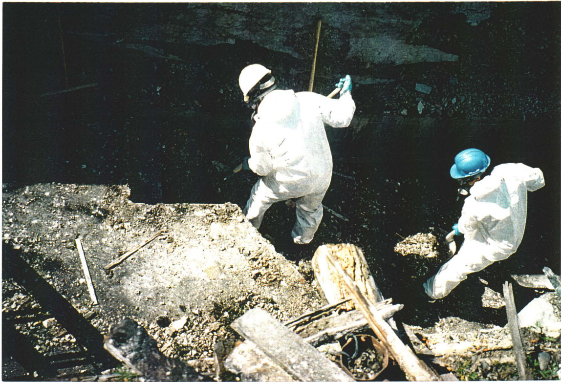
PHOTO 1: Barracks Building - Manual removal of moss and debris indicated by ESG (ESG 1995) to contain concentrations of PCBs above CEPA criteria.
