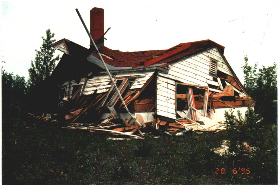
Photograph III-3: The Tower Building as it appeared in July 1995, before the start of remediation activities in June 1996.
