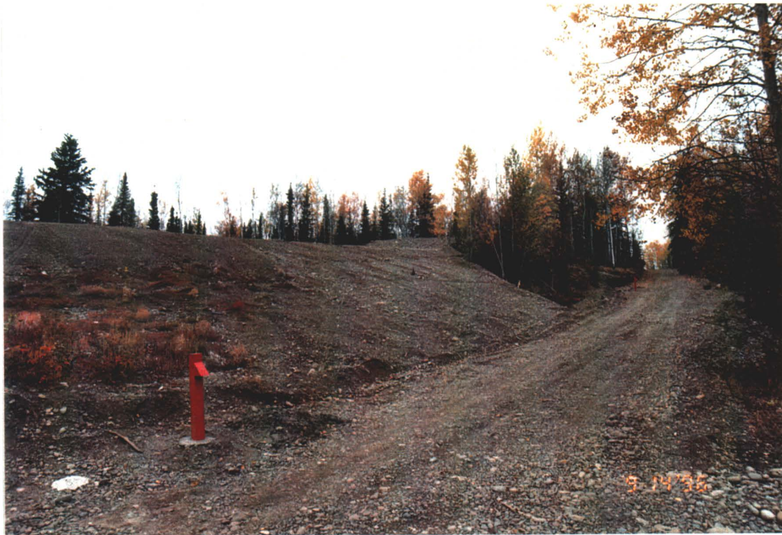
Photograph IV-5: The Snag Airstrip Dump, after the application of additional fill and regrading, and the installation of monitoring wells.
