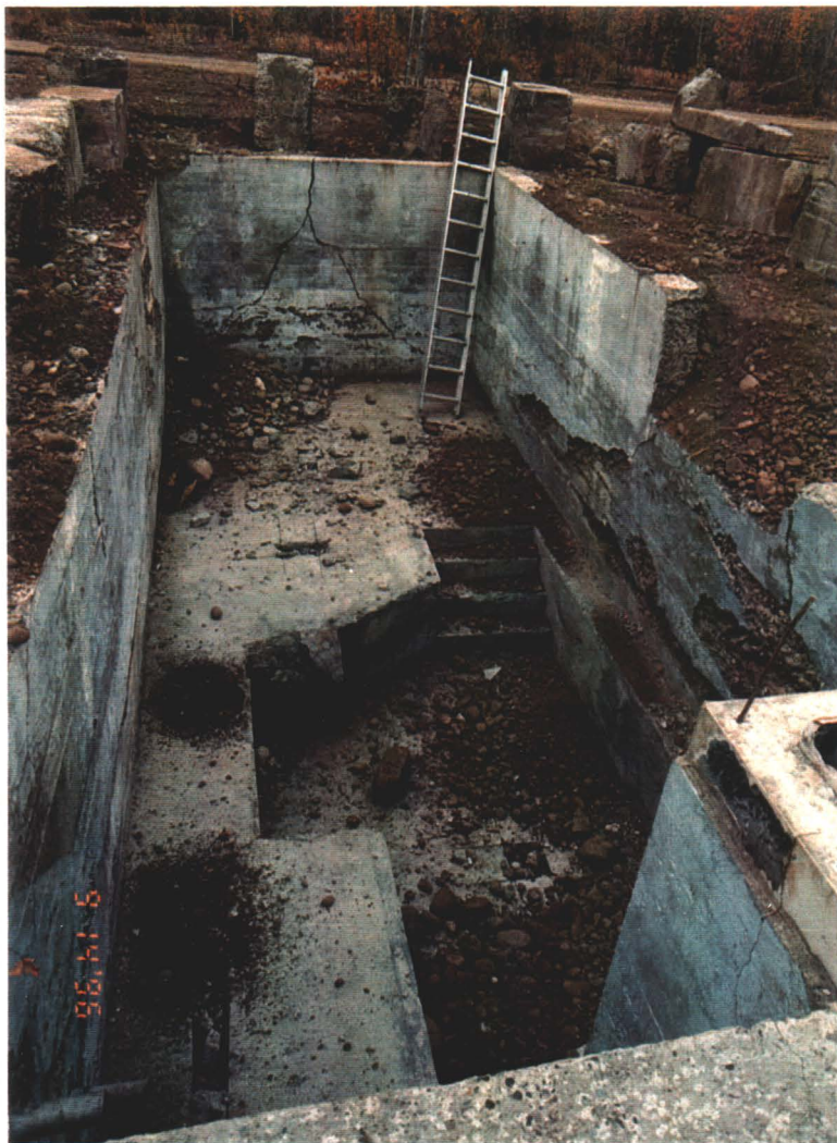
Photograph IV-3: The DOT Barracks Building basement following containerization of debris and moss contaminated with PCBs and dioxins. In addition, a portion of the foundation was later containerized because high levels of PCB contamination were detected in the cement.
