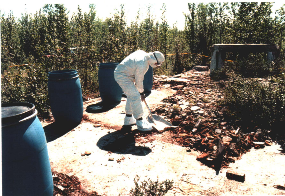
Photograph III-11: Removal of PCB-contaminated surface debris from the Powerhouse Foundation was completed by the ESG field team.
