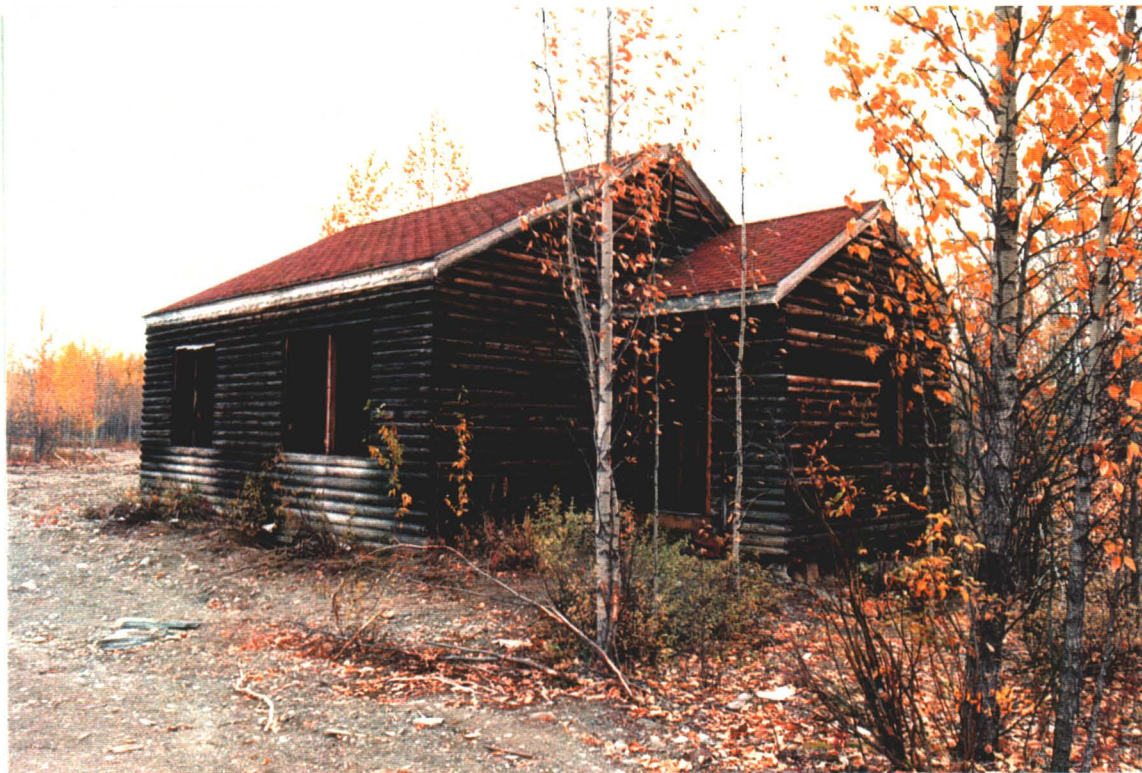
Photograph III-15: The exterior of the Married Quarters after all interior materials with painted surfaces were removed.
