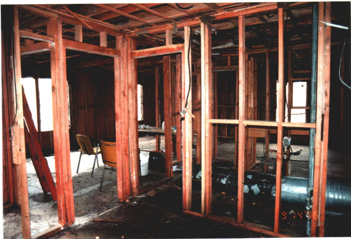
Photograph III-16: The interior of the Married Quarters following the removal of all interior materials with painted surfaces.
