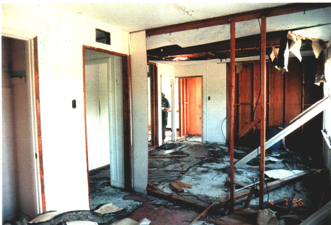
Photograph III-14: The interior of the Married Quarters had been vandalized over the years prior to the cleanup.
