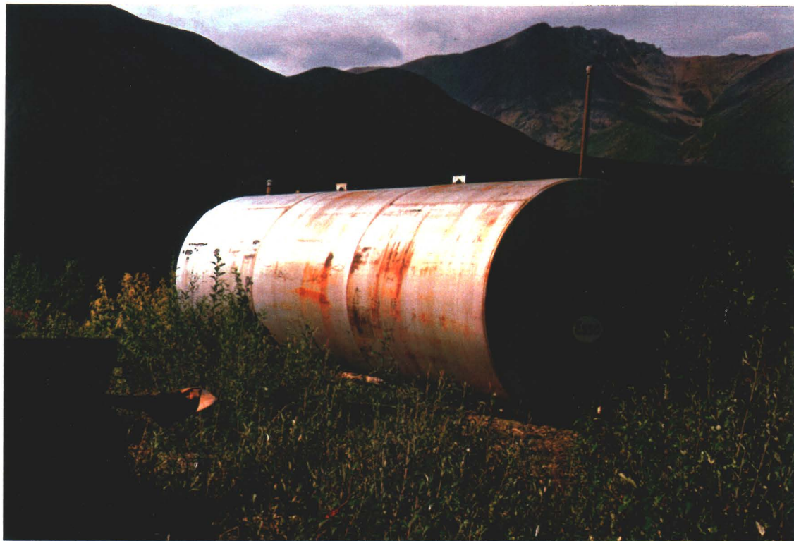
Photograph # 10: Storage tank ST - 1, contains 5,200 litres diesel fuel.
