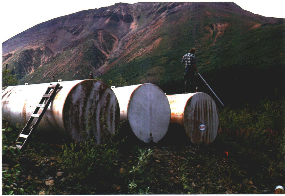
Photograph # 16: Storage tanks TC - 8, 9, and 10. Contain 14,900 litres spoiled gasoline.
