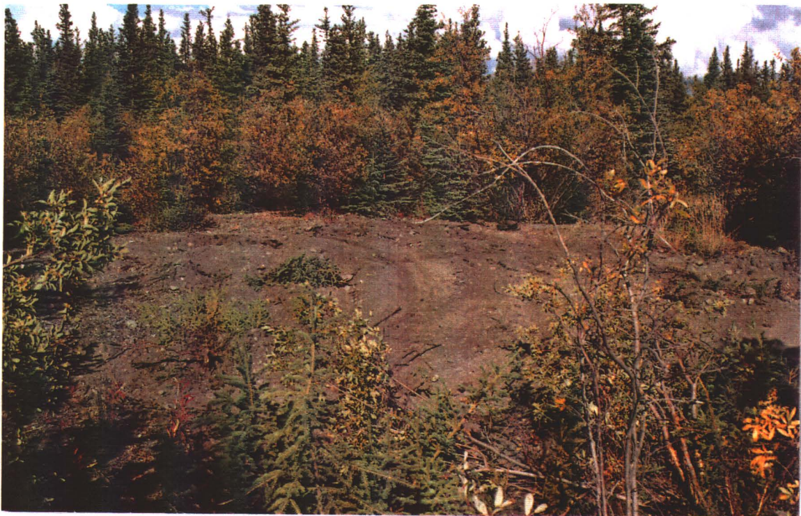
Photo 8 Final Excavation #7 - Northwest corner of property. No buried drums were located in this area. Soil staining was evident. ( See Analytical Results)
