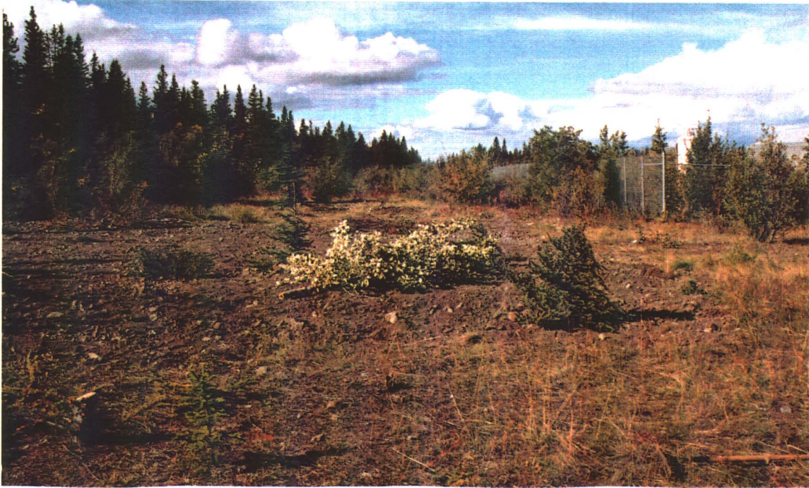
Photo 5. Excavation #1 - Southwest of main building. No buried drums were located in this area.
