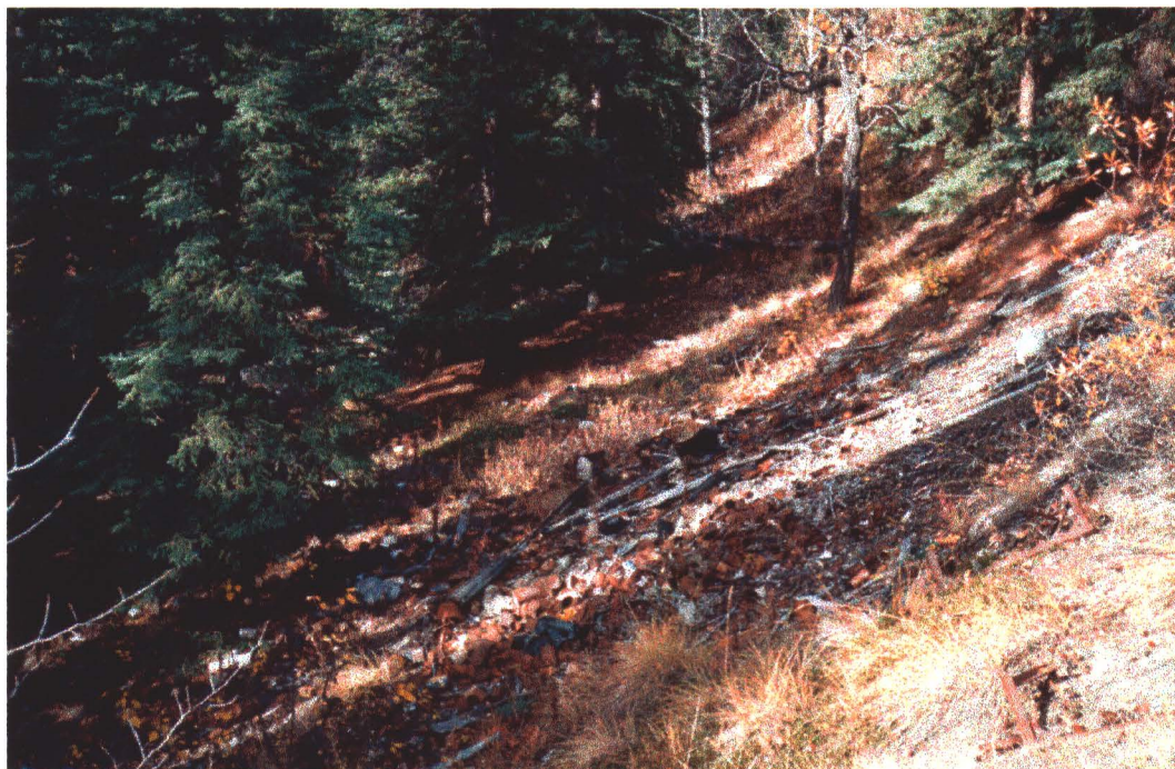
Photograph 16 - Mendenhall River - Surface debris on slope.
