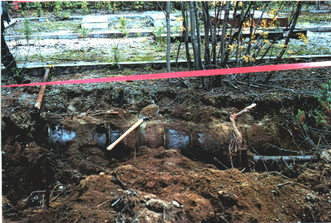
Underground storage tank located on west side of large foundation.
