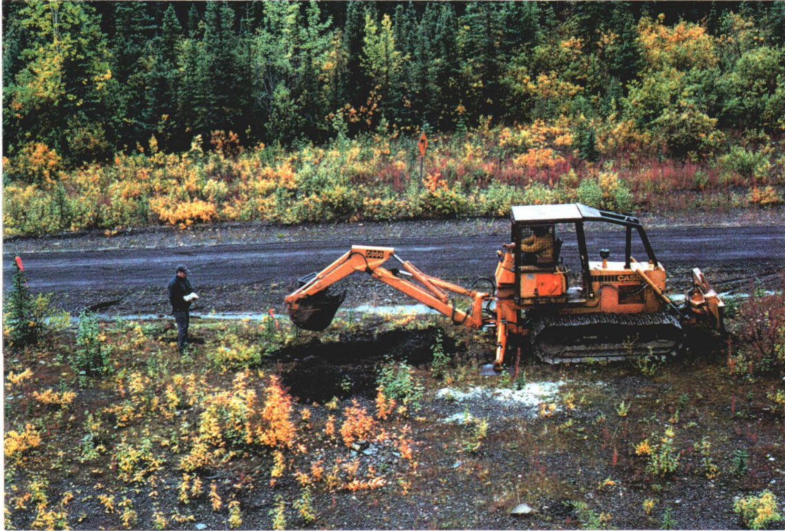
Test pitting soils along north side of Canol Road. Looking south from top of rock face.
