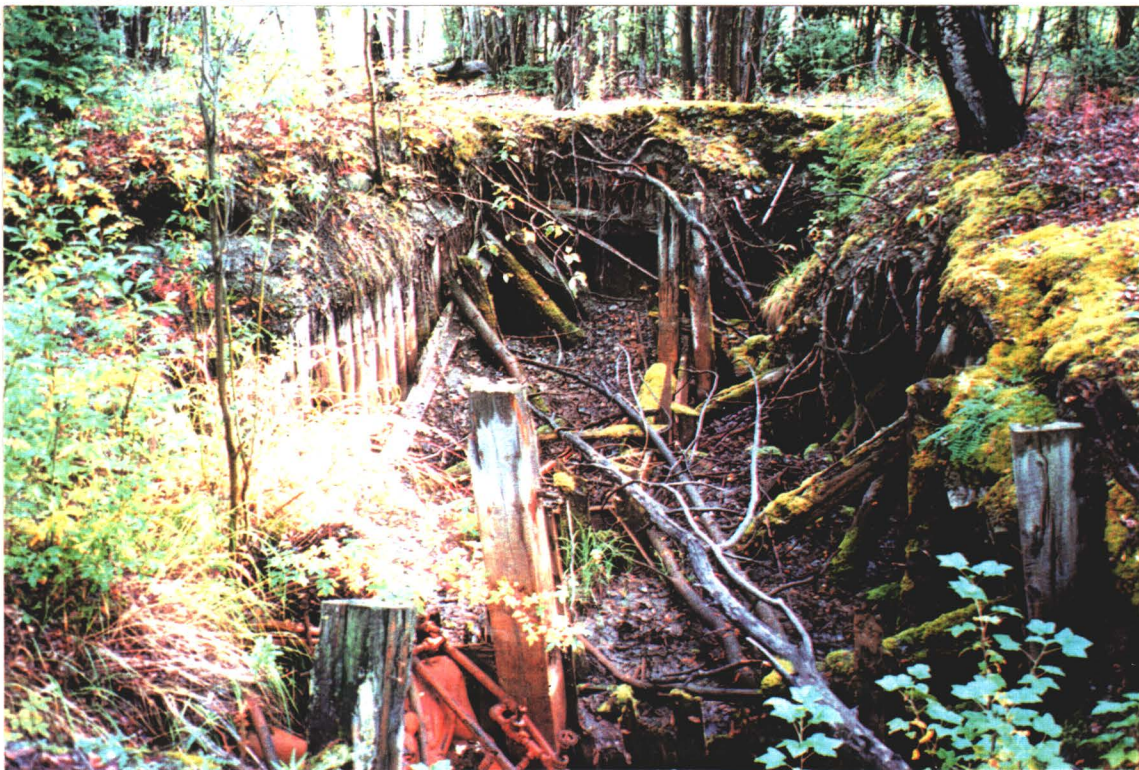
Collapsed wood frame pit on east side of road.
