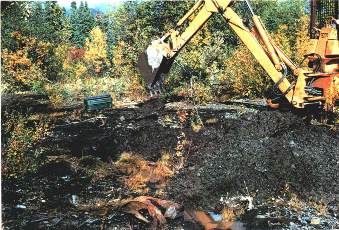
Excavating test pits in impacted areas. Note crushed drums on surface. These were encountered while digging.
