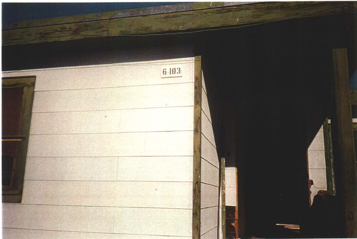
Single Residence. Note white asbestos cladding.
