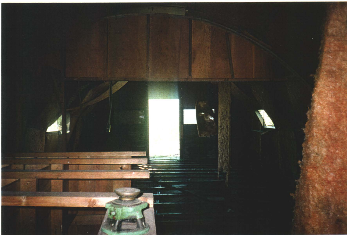
Interior of Quanset. Extensive vandalism. No asbestos.
