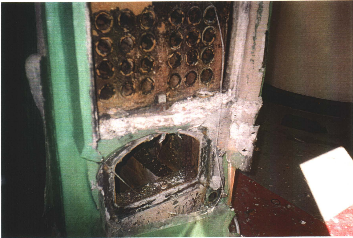
Multi-family Dwelling, Boiler Room. Boiler and tanks present. Friable asbestos present in abundance due to vandalism. Very hazardous conditions.
