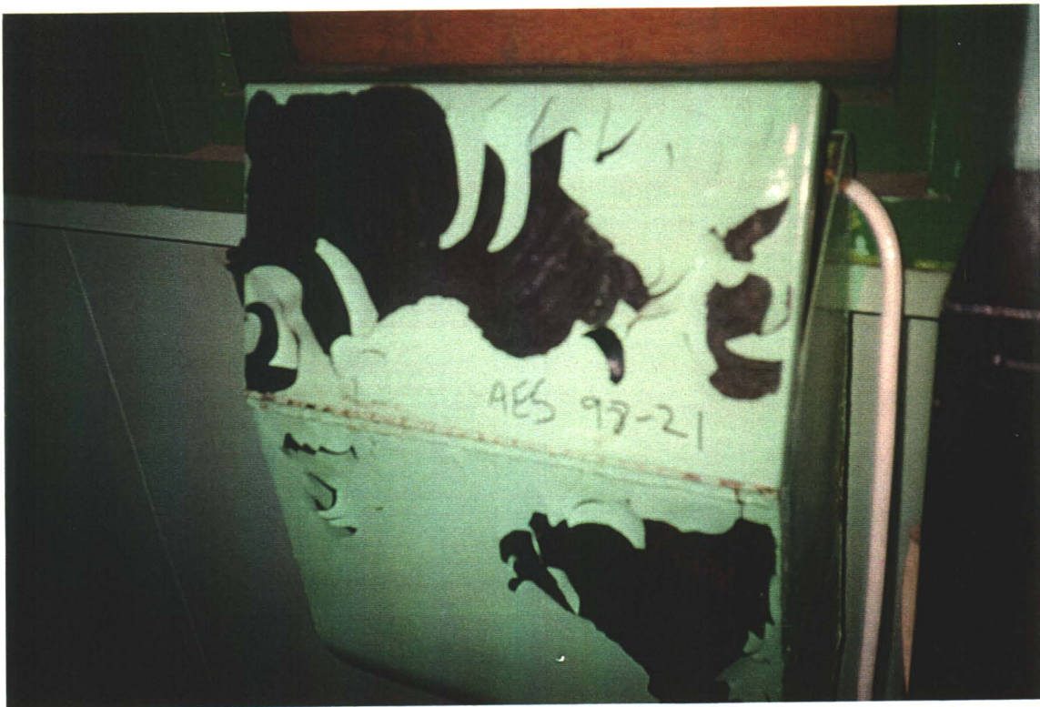
Compressor Building. Flaking green lead-based paint common to all equipment components.
