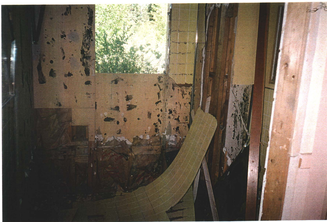
Single Residence. Note extensive vandalism.
