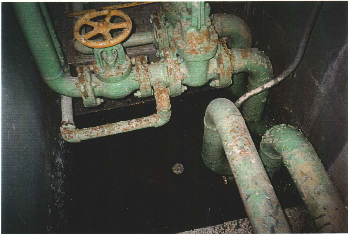
Compressor Building, Engine Room. Pit below engines. Contains water only. No environmental concern.
