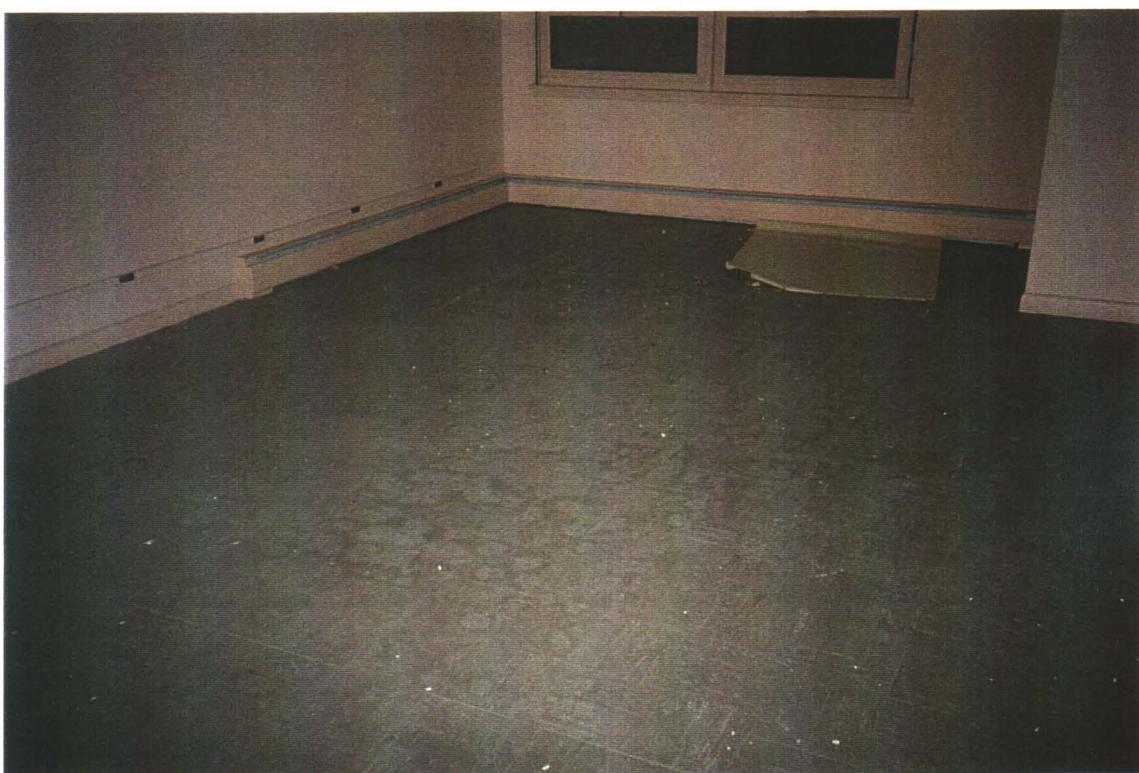
Multi-family Dwelling, living room. Note asbestos floor tiles.
