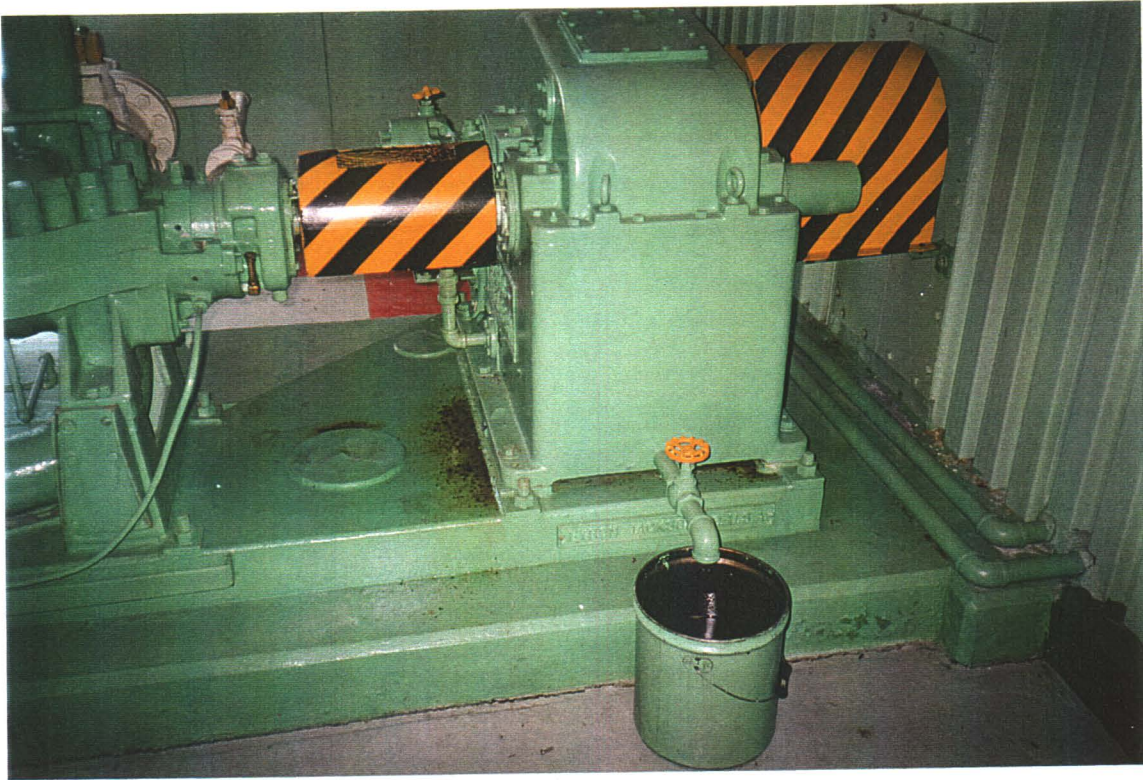
Compressor Building. Pump unit. Note fluid drained from mothballed unit.
