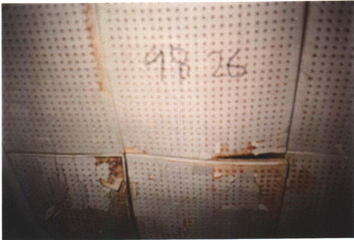
Compressor Building, Office Room. Sample from ceiling tile confirms no asbestos content.
