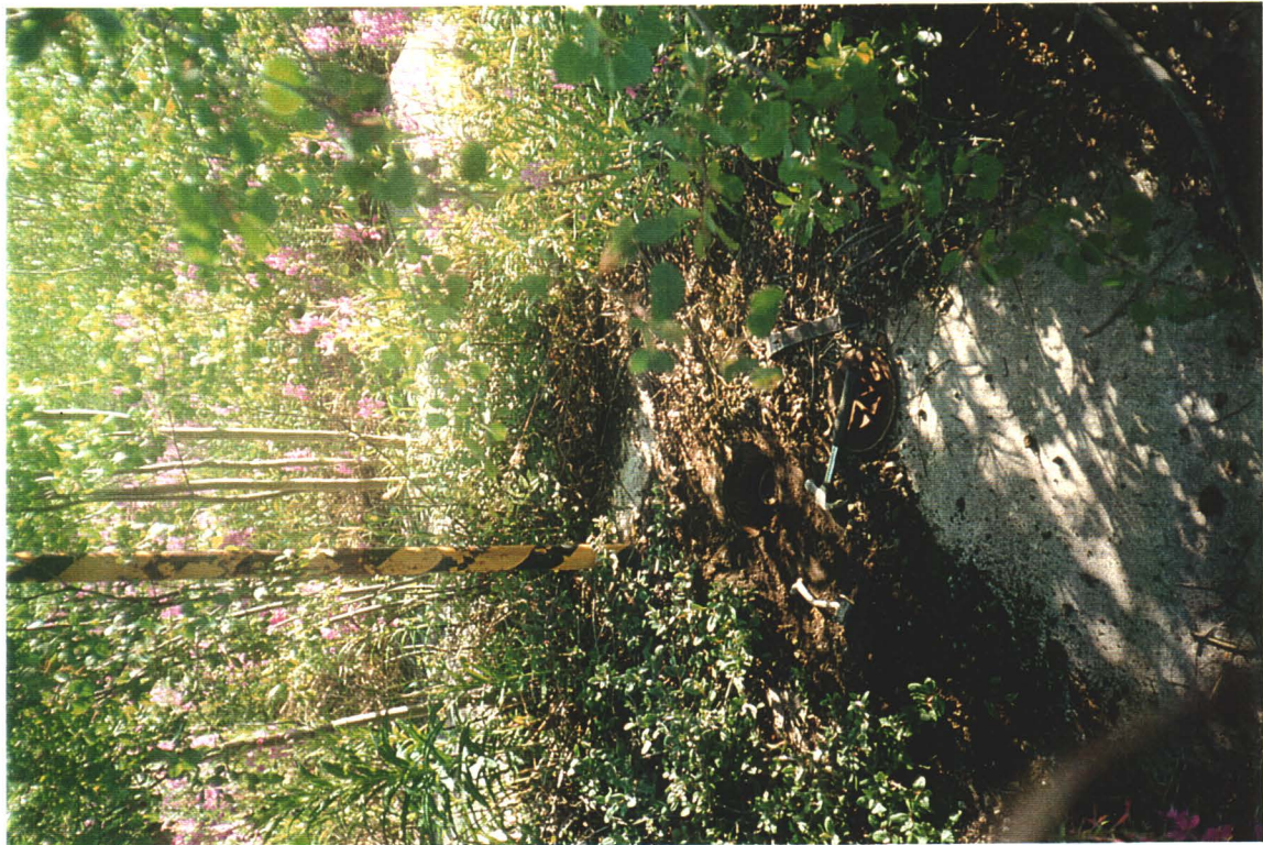
Concrete underground storage tank(s) for vehicle fuel.
