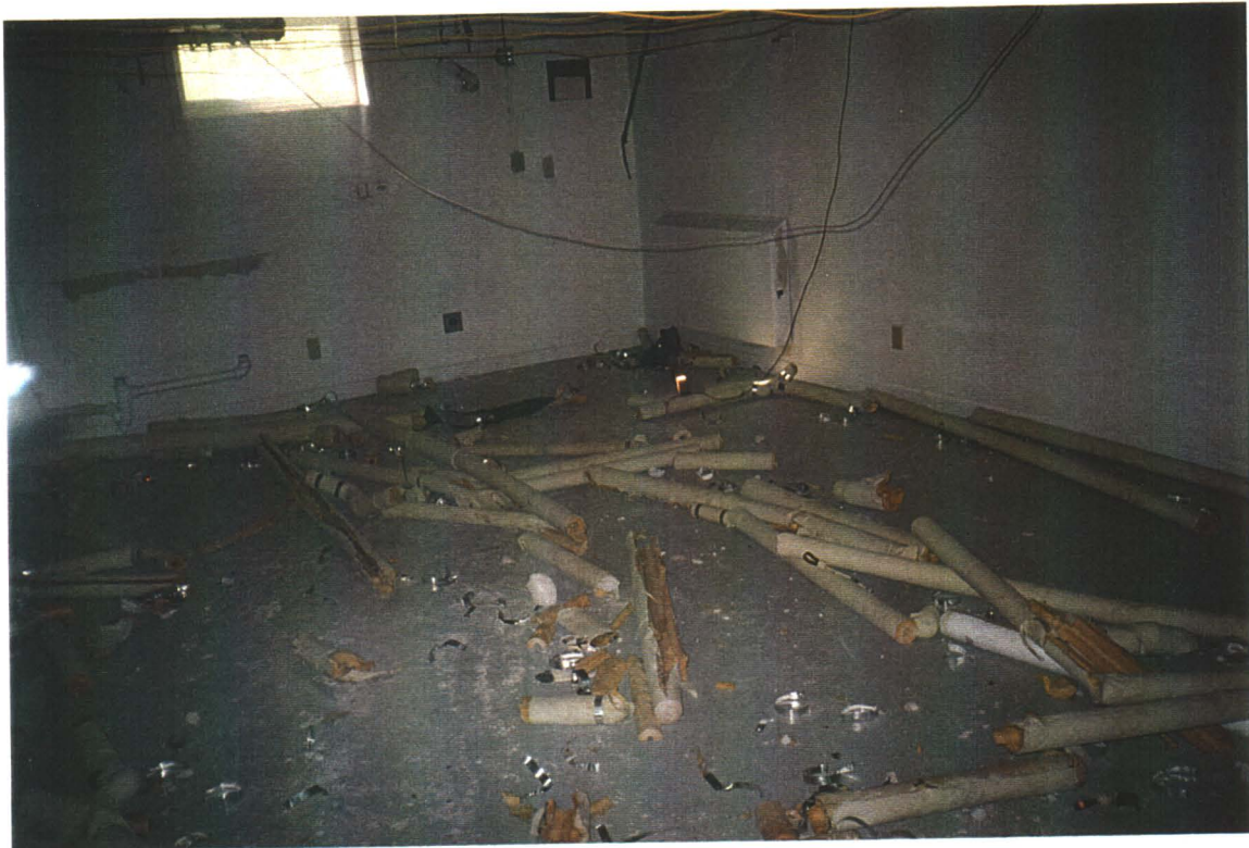
Multi-family Dwelling, basement. Note extensive vandalism, including exposure of asbestos containing materials (knuckles only) in pipe insulation. This has created hazardous conditions throughout the building, as asbestos fibres move with the airflow.
