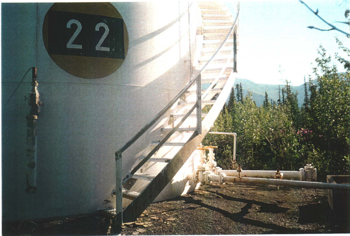
Bulk fuel storage tank, 1 of 2. Empty.
