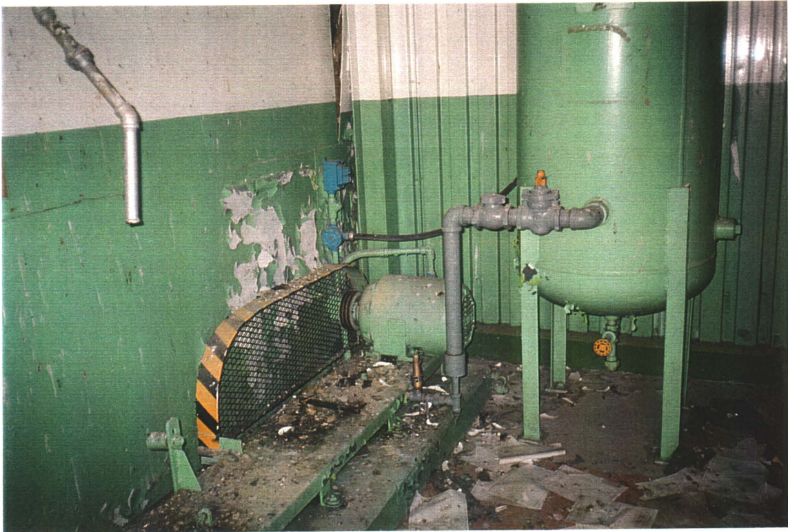
Compressor Building, Engine Room. Small compressor unit gone, but 3 phase motor and pressure tank remain.
