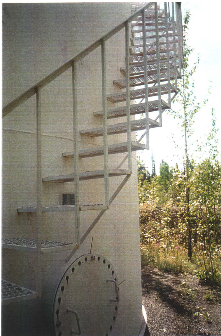
Main product tank, 1440 barrel capacity. Man-way loosely bolted, indicating entry following product removal.
