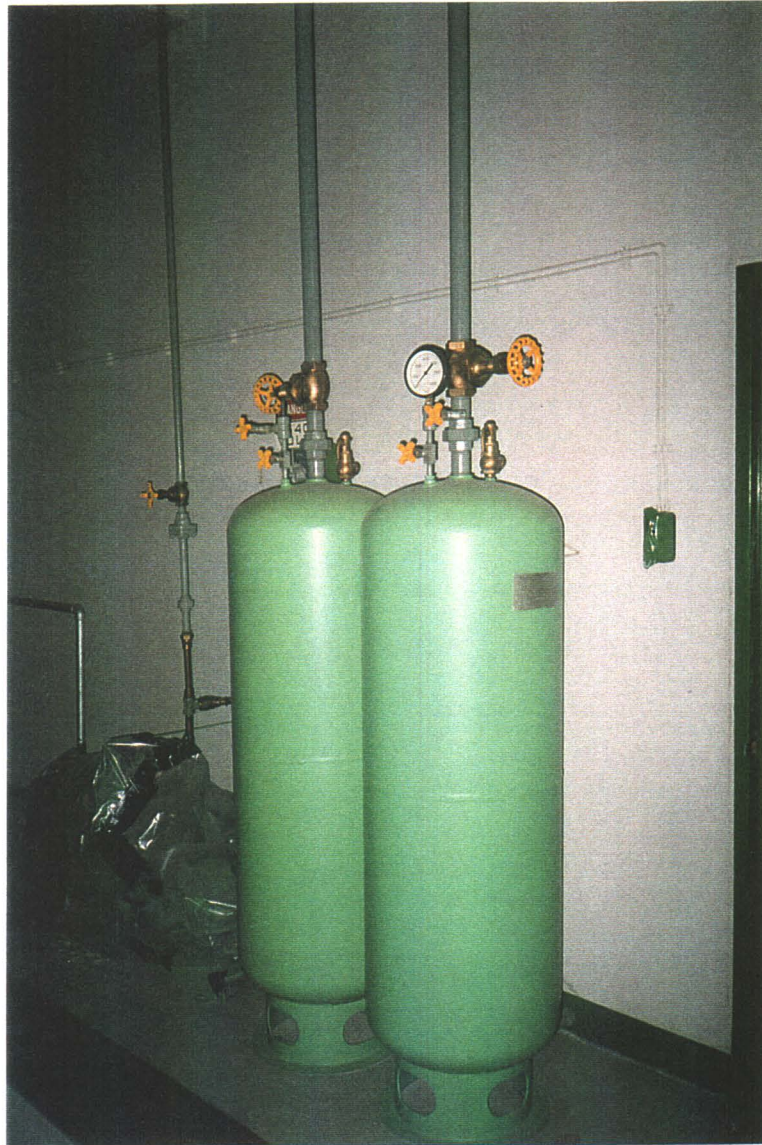
Generator Room. Compressed gas vertical storage tanks, currently drained.
