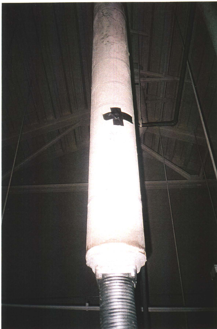
Generator Room. Generator stacks confirmed to contain friable asbestos (sample 98-12).
