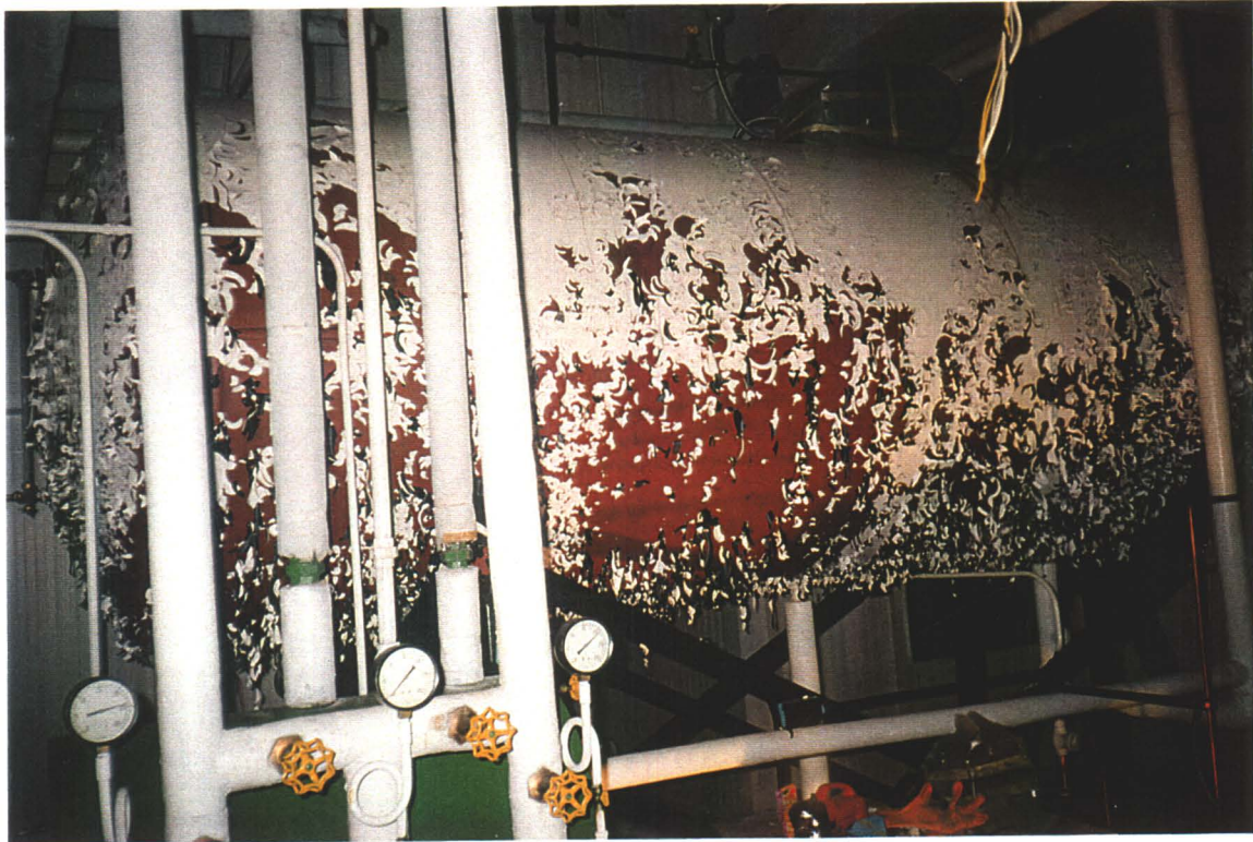
Boiler Room. Water storage tank, completely drained. (note: lead based paint is flaking off)
