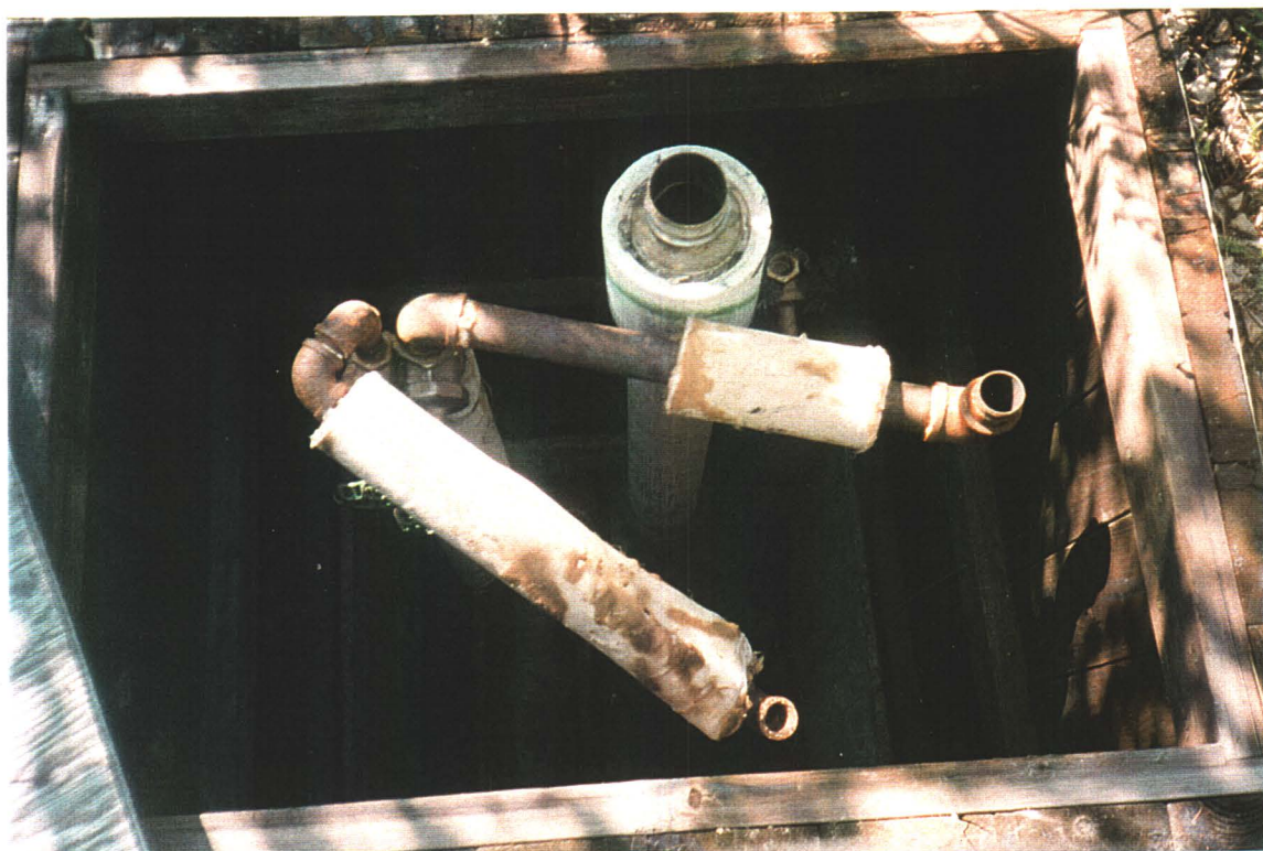
Typical services pit at each trailer stall (one of six). (Note: transite asbestos pipe sewer connection)
