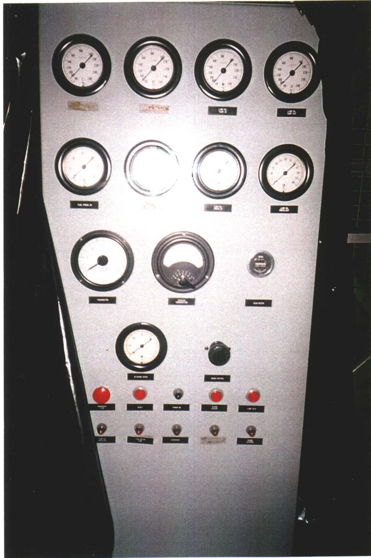
Engine Room. Engine control panel (one of two).
