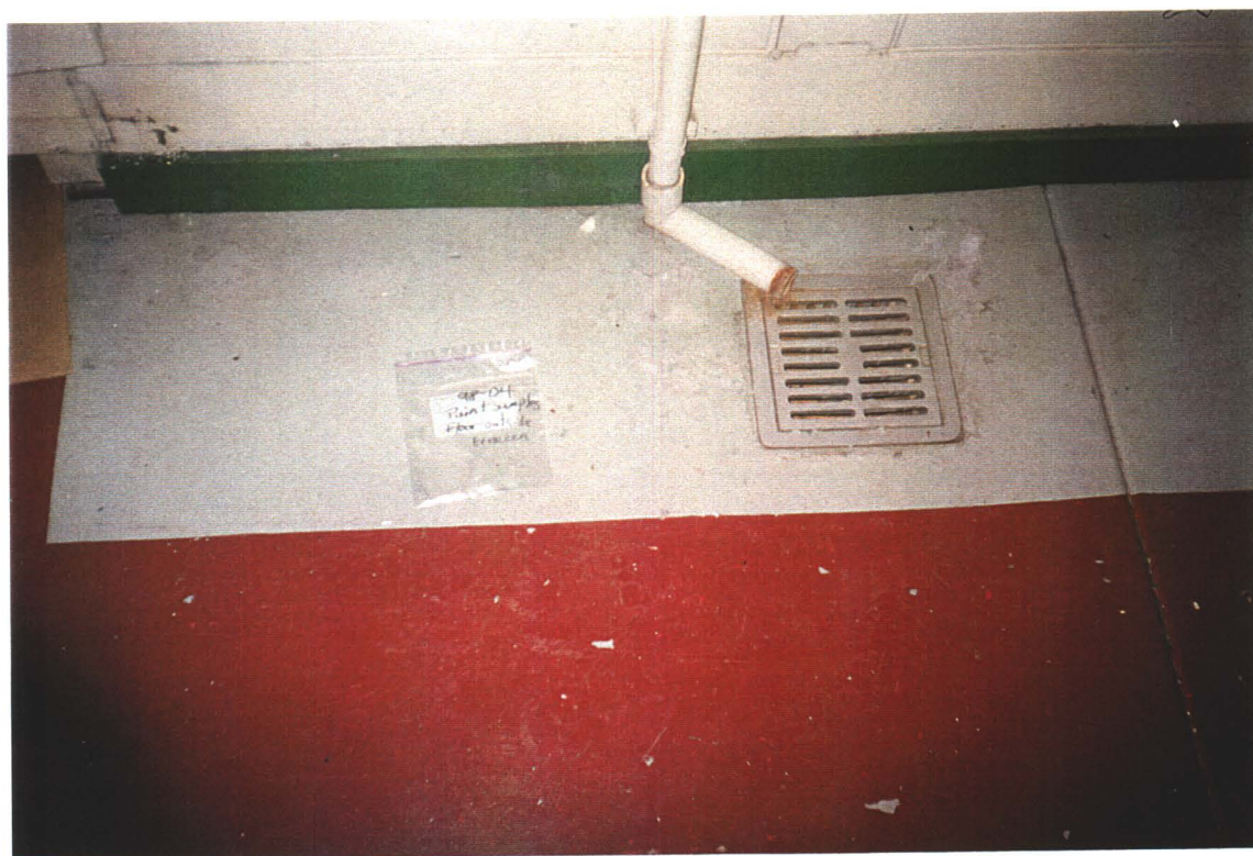
Store Room. Paint sample taken from floor in front of lockers. (Identified as lead-based paint)
