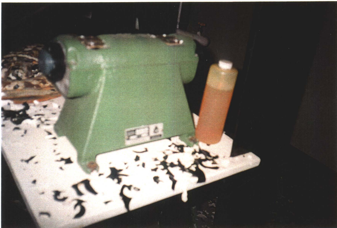
Boiler Room. Injection pump, for metering chemicals to water tank.
