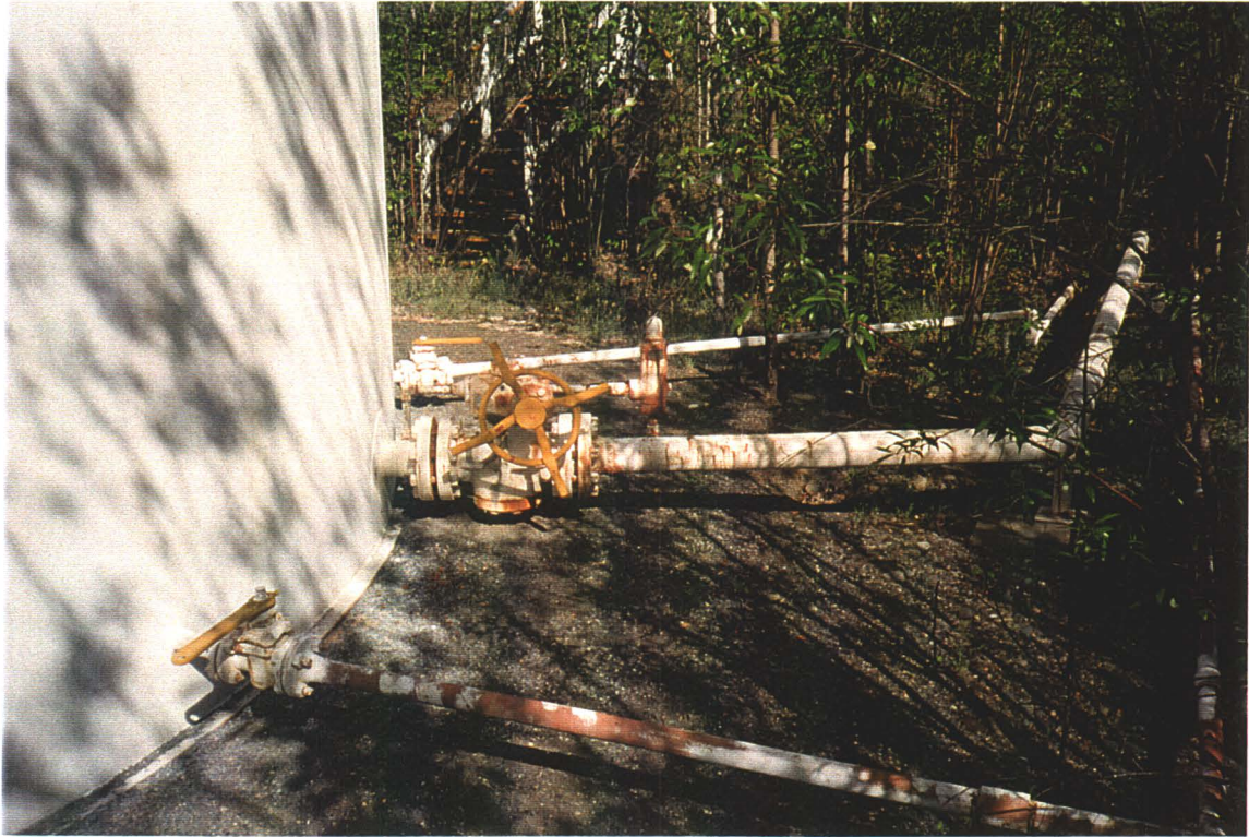
Bulk storage tanks line connections.
