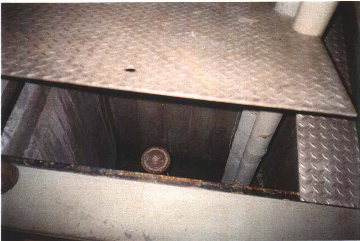
Boiler Room. Entry for underground conduit.
