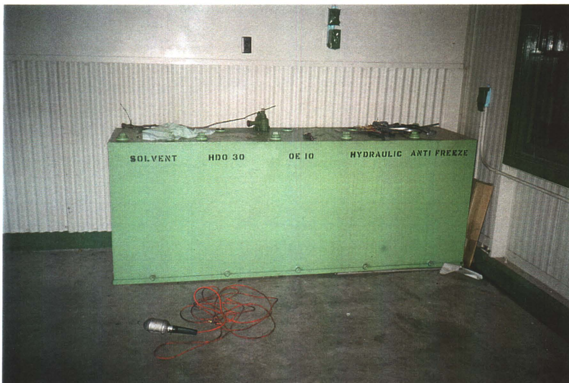
Mechanical Room/Shop. Maintenance fluid storage tank. (Note: there are about four inches of product in each separate compartment)
