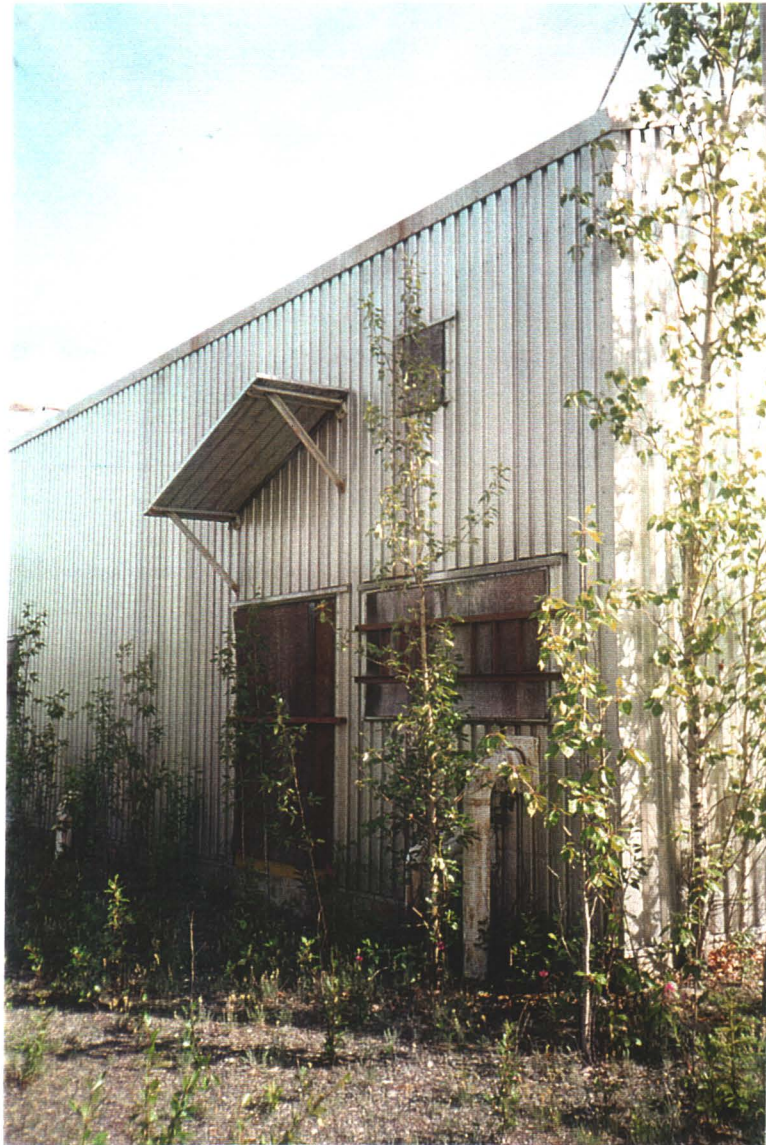
Main Building. Pipeline entry/exit lines.
