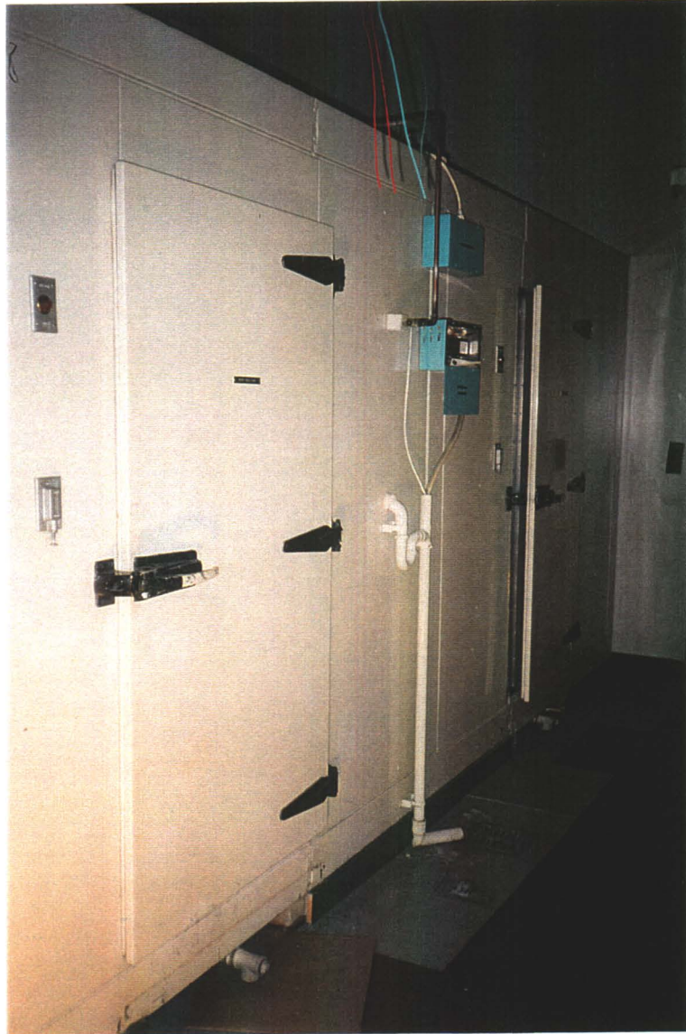
Store Room. Side by side walk-in cooler and freezer units. These units are complete, and are likely charged with coolant
