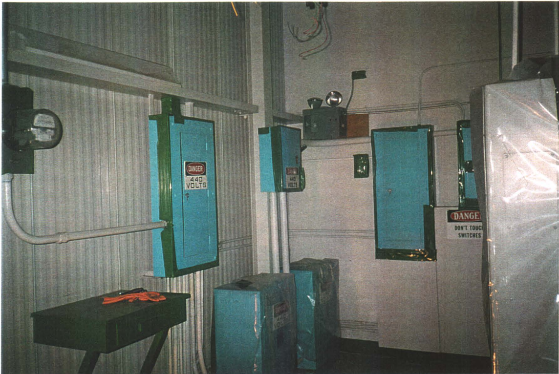
Generator Room. Sealed power panel boxes. Note 440 volts/3 phase power supply, and dry transformers
