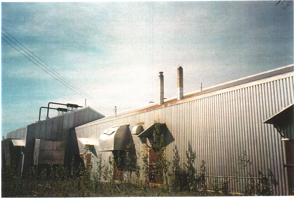
Back of main building. Note stainless steel ventilation structures, and asbestos-filled Generator Room stacks.
