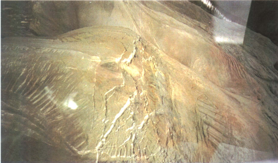
UMA Photo 3-13: Tension cracking of Upper Slope (1998)
