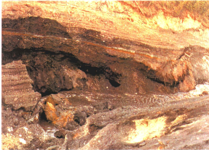
Photo CC-09: Erosion of Access Road on North Side of Creek (1975)
