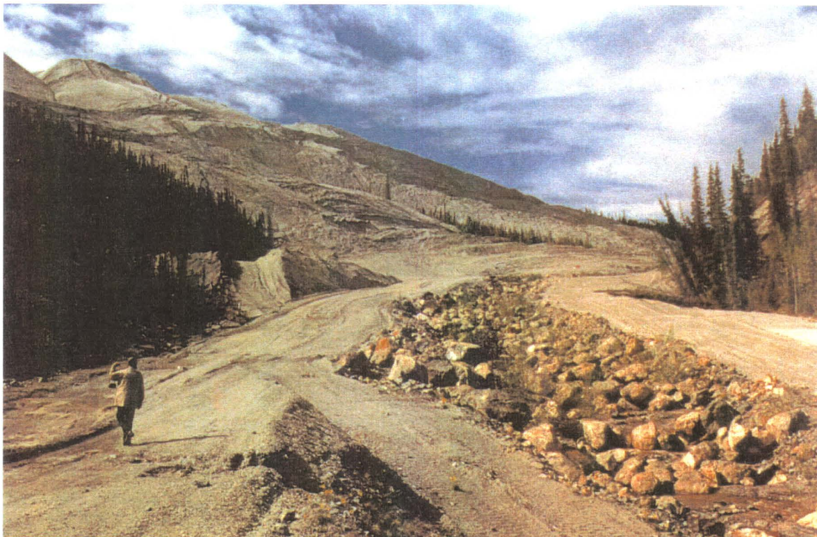
Photo 22: Armouring of Wolverine Creek Channel Downstream of the South Lobe
