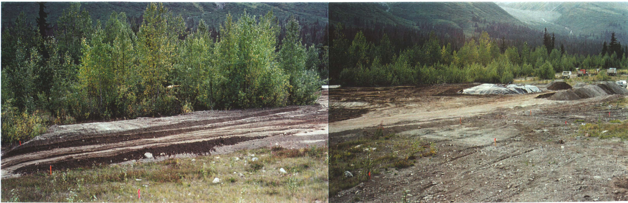
Photograph 1: Border Station showing the partially placed cap at the former location of the Temporary Storage Facility, the stock pile of clean fill required to complete the cap, and tarp covering the temporary stock pile of contaminated soil excavated from DDT contaminated areas.
