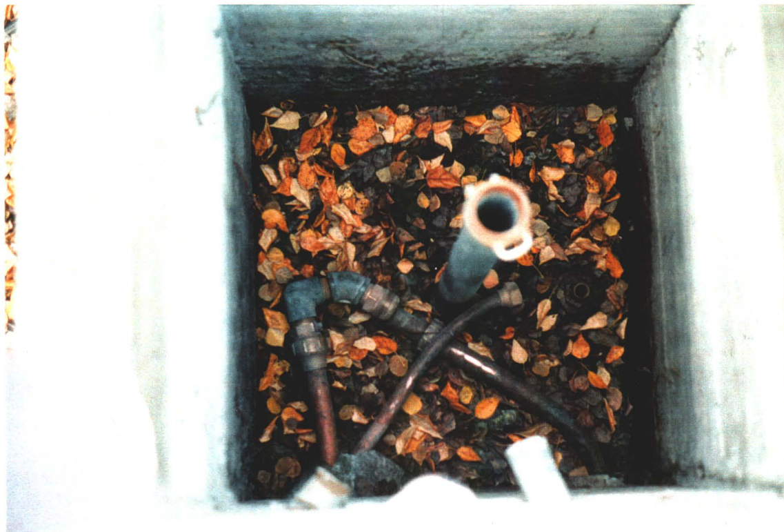
Concrete well with copper fuel lines.
