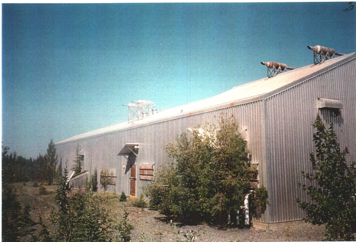
Main Building. Pipeline entry/exit lines.
