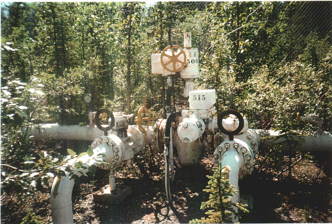
Bulk storage tanks line connections, back of Main Building.
