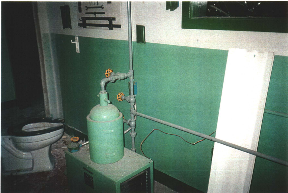
Engine Room. Compressor air intake filter device.
