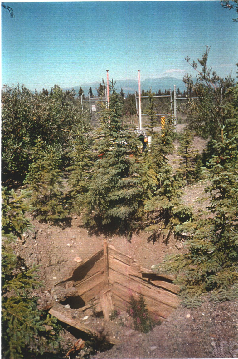
Pit area between bulk product tanks and UST's
