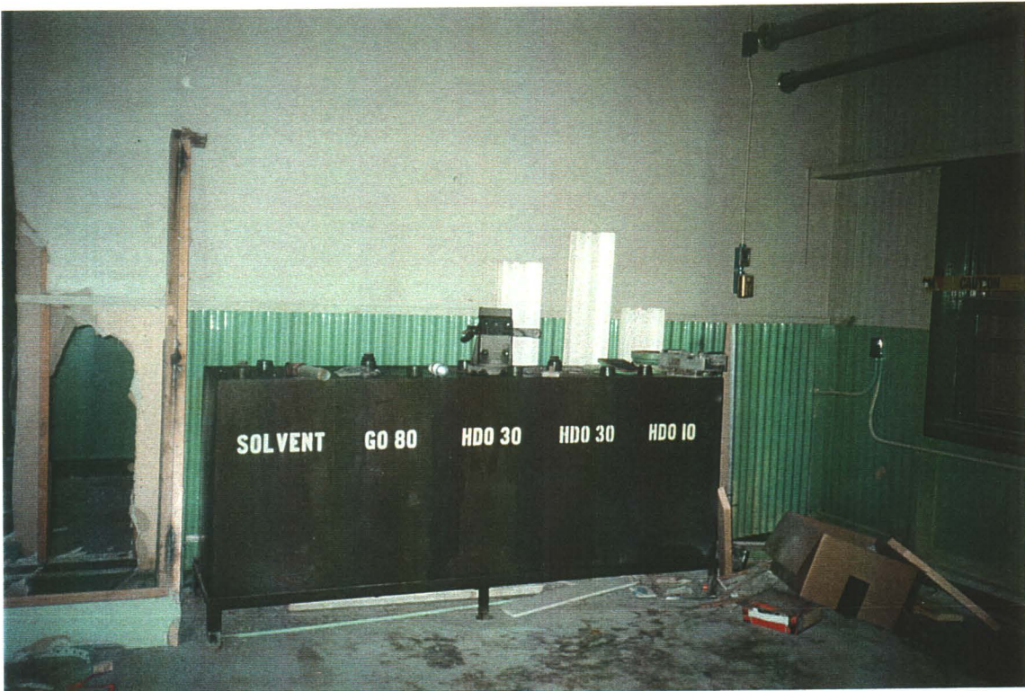
Mechanical Room/Shop. Maintenance fluid storage tank.
