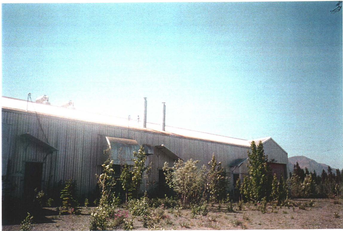
Front of main building. Note stainless steel ventilation structures, and asbestos-filled Generator Room stacks.
