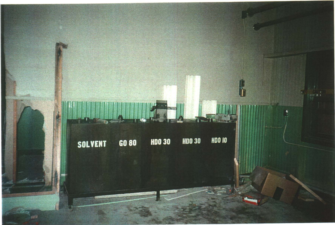
Mechanical Room/Shop. Maintenance fluid storage tank.
