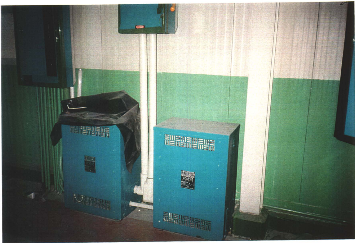
Generator Room. Transformers (dry type)
