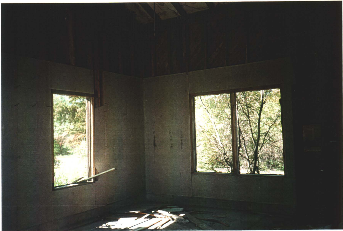
Pump House building interior. Note 5 sheets asbestos wallboard.
