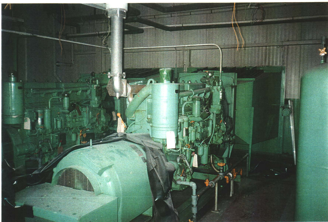
Generator Room. Generator Units. Stacks contain asbestos insulation.
