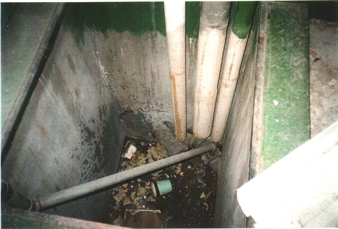
Boiler Room. Steam, sewer, and water lines leading out to former housing area. Condensate return line returns back to boiler room.
