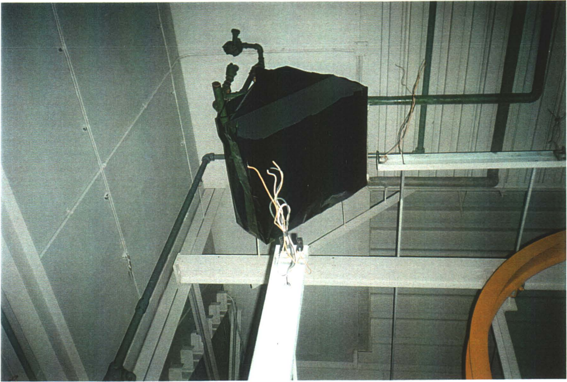
Engine Room. Typical overhead heater device used throughout the building.
