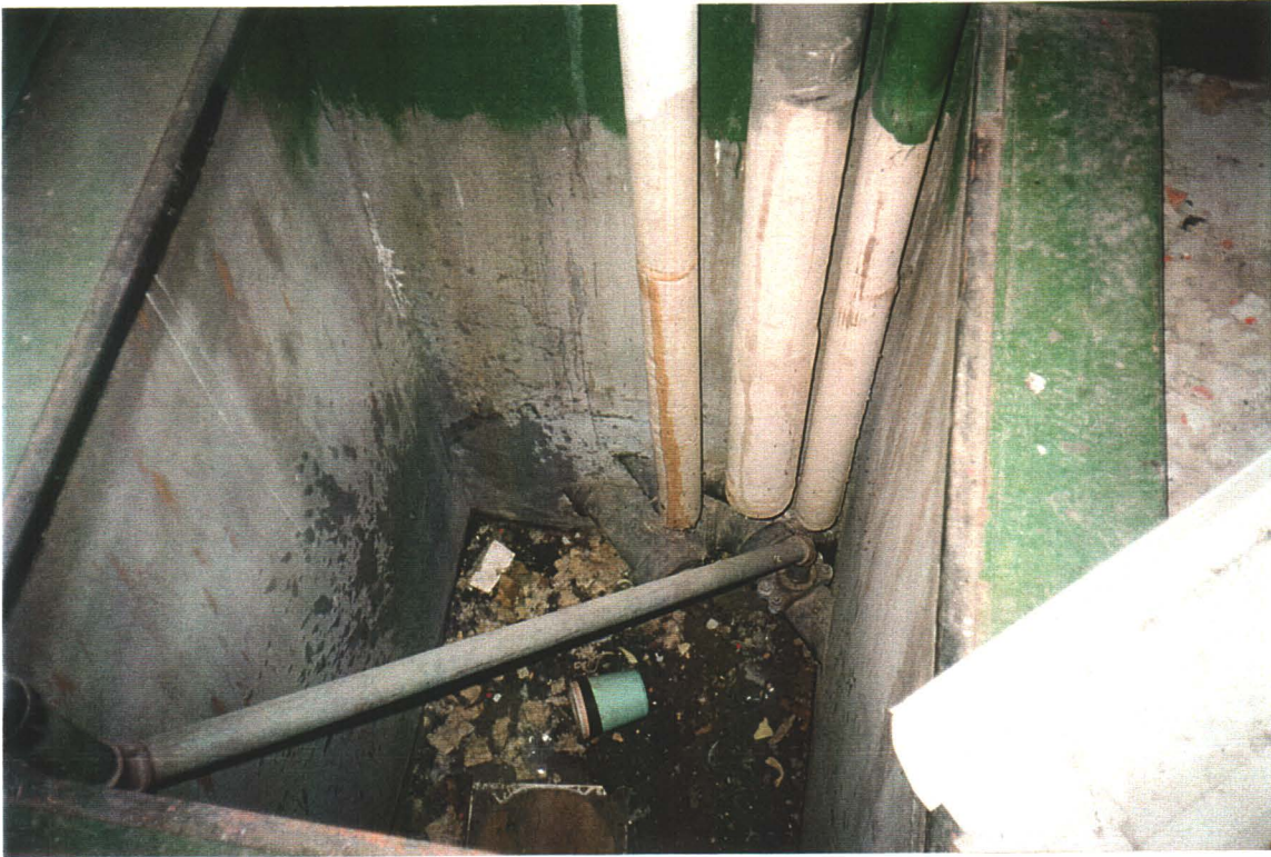
Boiler Room. Steam, sewer, and water lines leading out to former housing area. Condensate return line returns back to boiler room.
