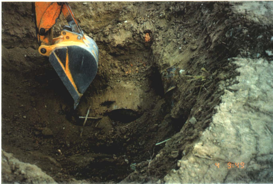
Plate 10 0N 28W Drums D2, D-3, sludge D-4 from this pit # 20
