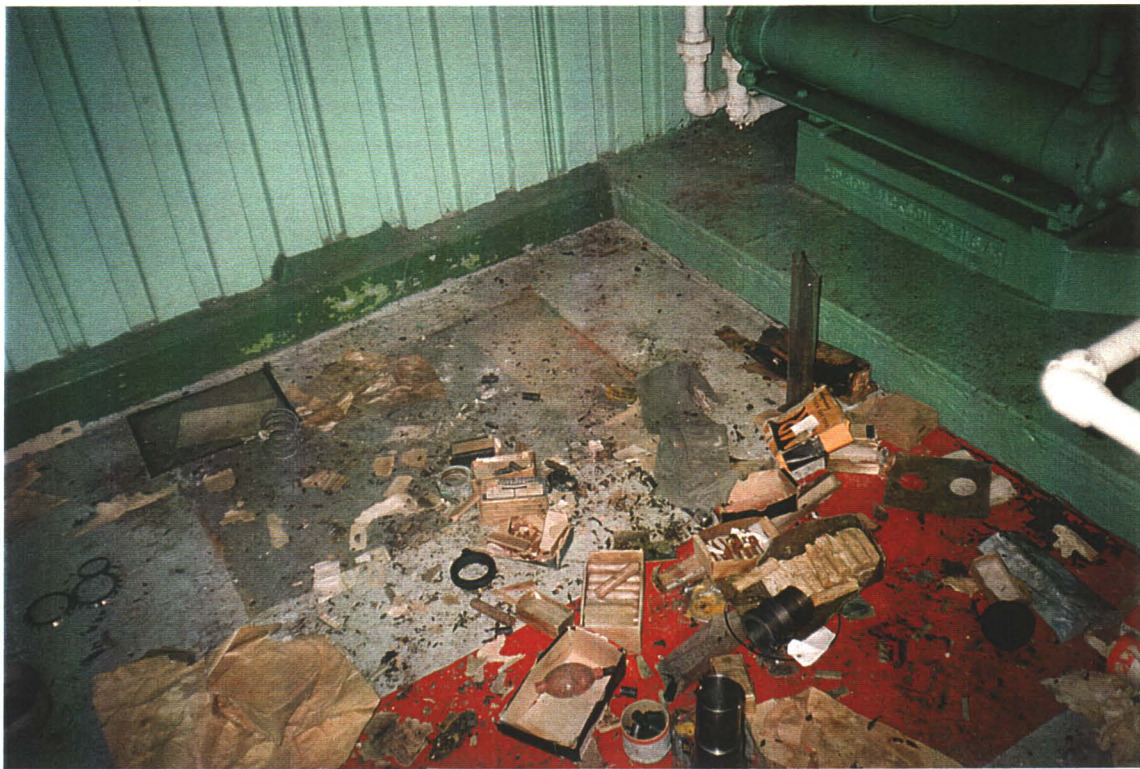
Compressor Building, Compressor Room. Debris on floor indicating vandalism
