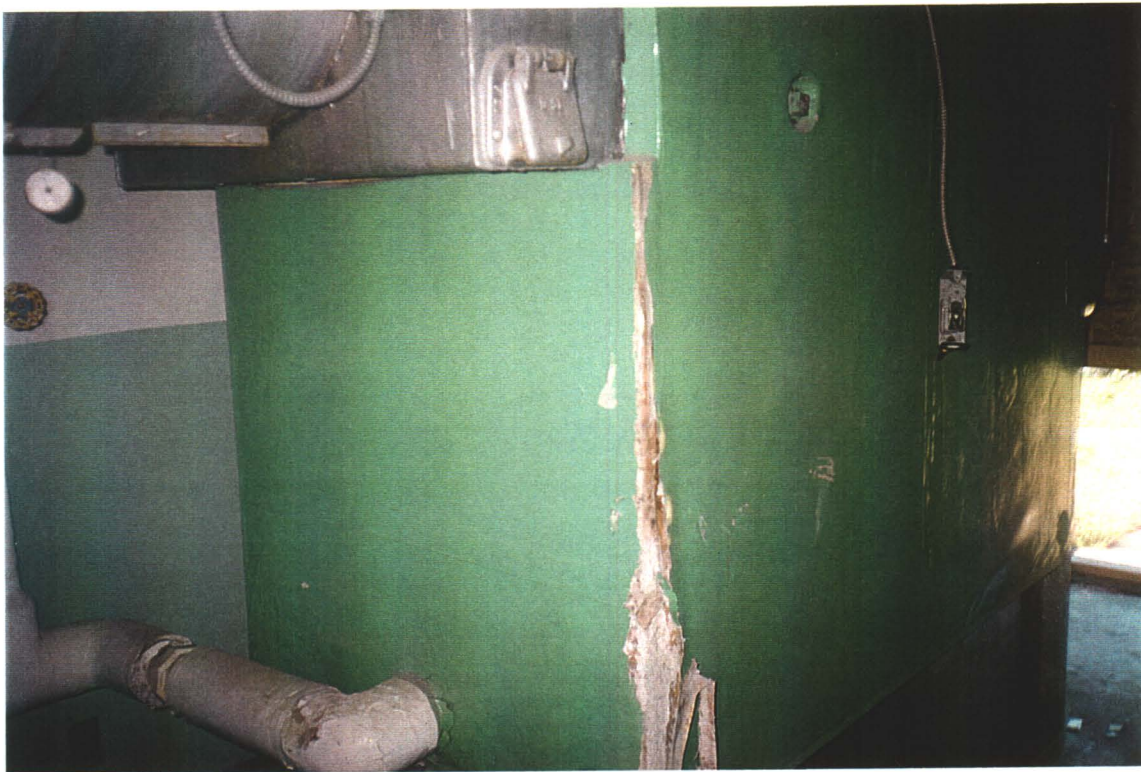
Multi-family Dwelling, Boiler Room. Boiler and tanks present. Friable asbestos present in abundance due to vandalism.
