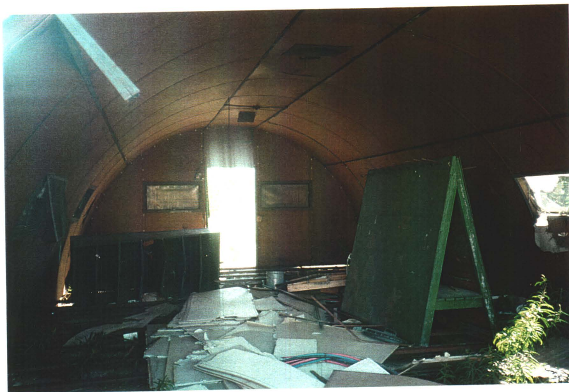
Interior of Quanset. Extensive vandalism. No asbestos.
