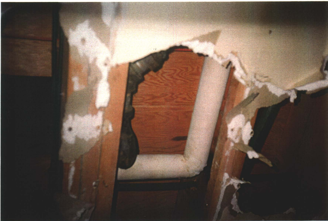
Multi-family Dwelling. Note asbestos knuckles in exposed heating pipes behind walls.
