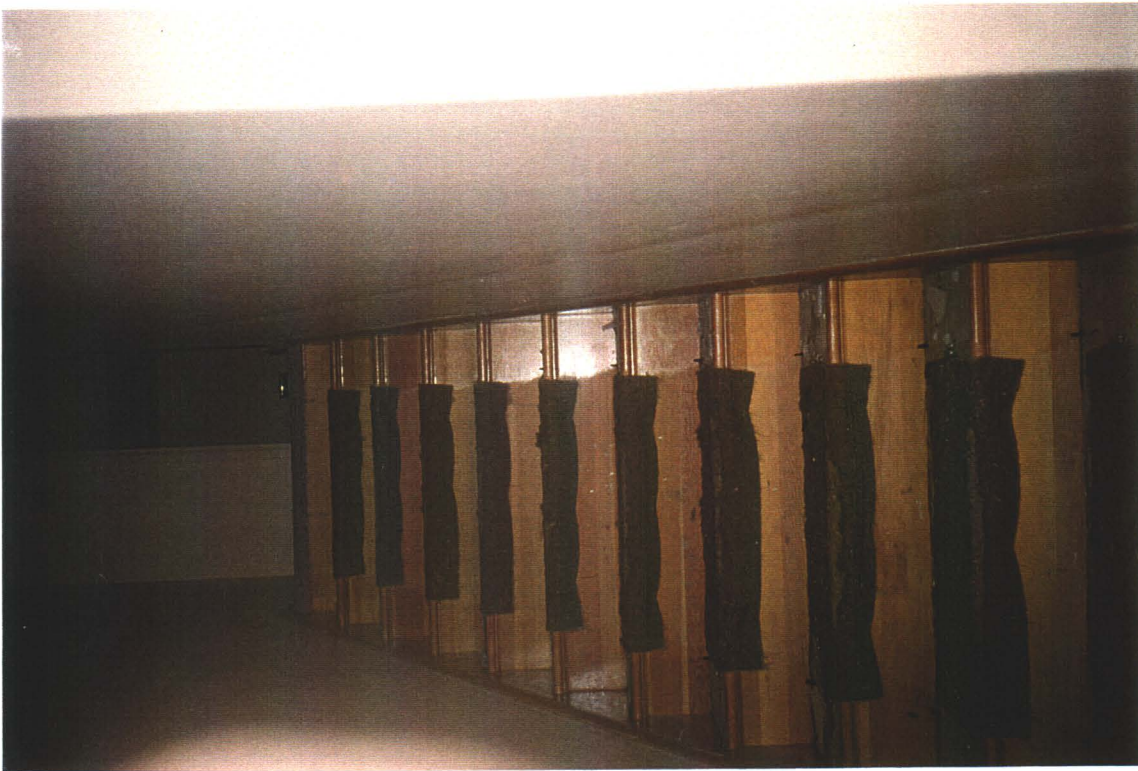
Multi-family Dwelling, interior stairway to second floor. No asbestos present, except for knuckles in heating system pipes, which are inside walls, and 9" x 9" floor tiles.
