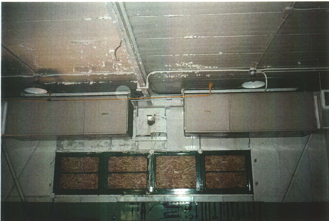
Main Building, Shop. Overhead heat exchanger. Note lead paint peeling from metal walls on building interior.
