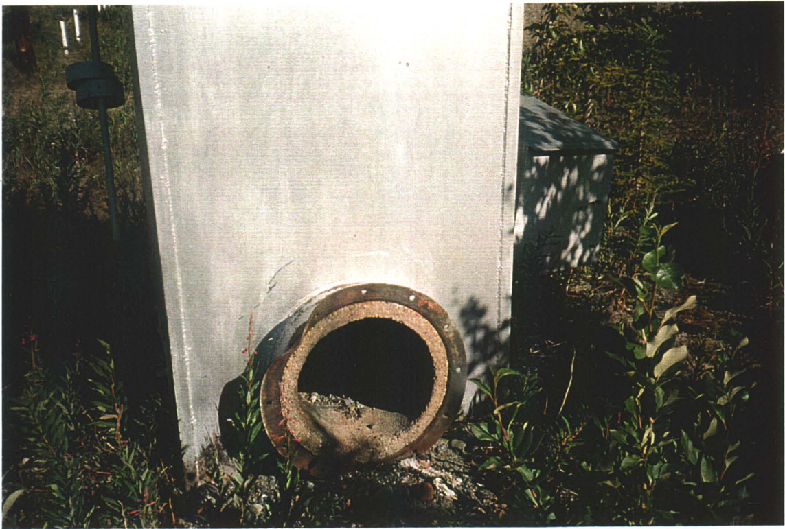
Garbage incinerator ceramic liner.
