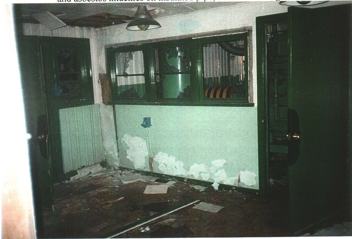
Compressor Building, Office Room. Ceiling material is asbestos free, whereas floor tile contains asbestos.
