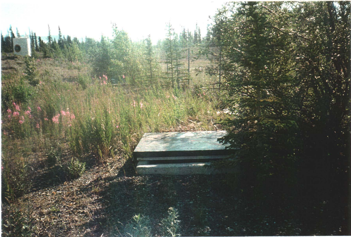
Sewage system vault array.
