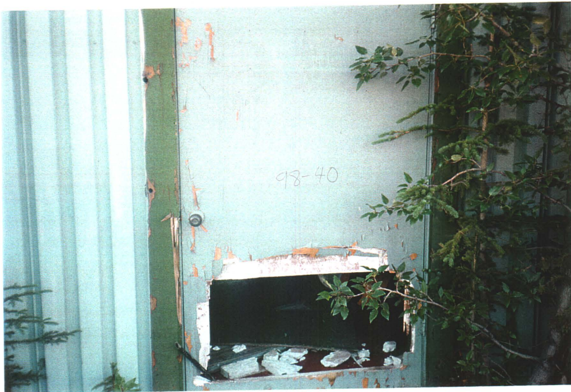
Compressor Building. Doorway to outside. Note that it has been kicked in, and that friable asbestos contained inside is now contaminating the Compressor Room
