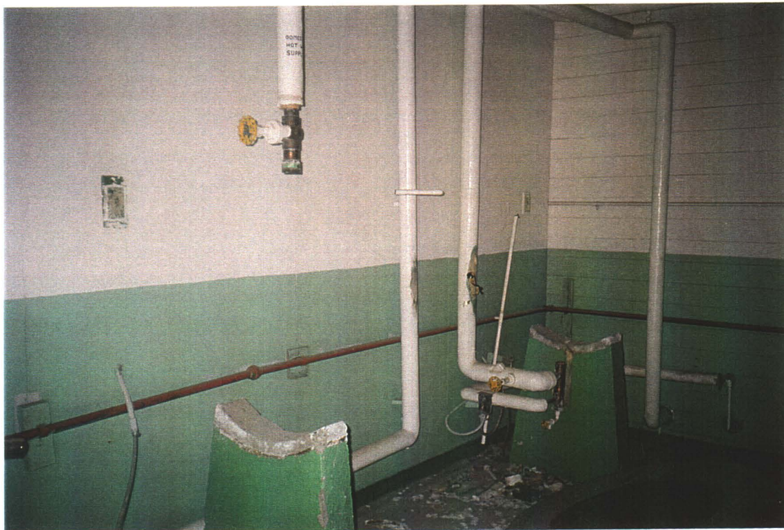
Multi-family Dwelling, Boiler Room tank is missing.
