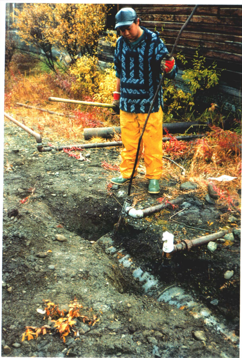
PHOTOGRAPH 9: Underground Storage Tank – Greg McLeod dips to check oil level – not oil on stick.
