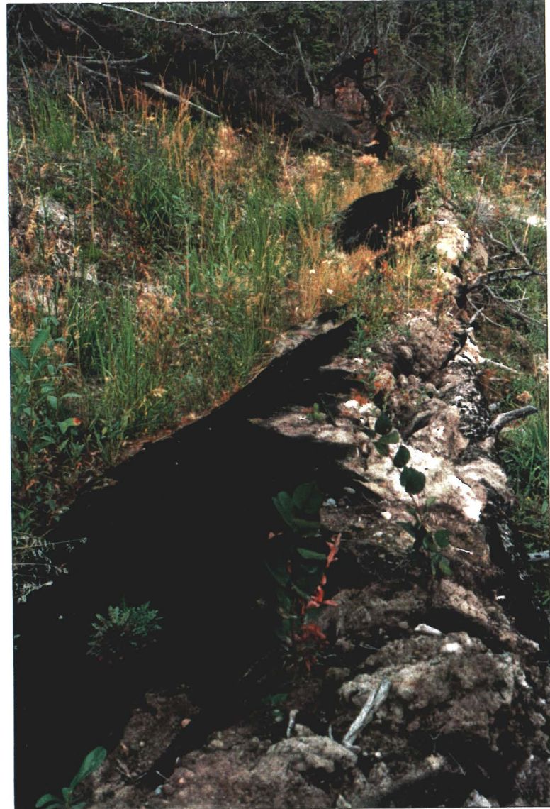
Photograph 4: Merrice Creek Sample Area #1. Geo-textile barriers on hill sloping south of site.
