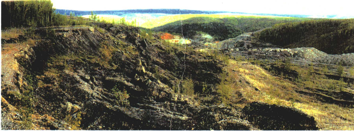
Photo 11: Crest of Unstable Waste Rock (1988)
