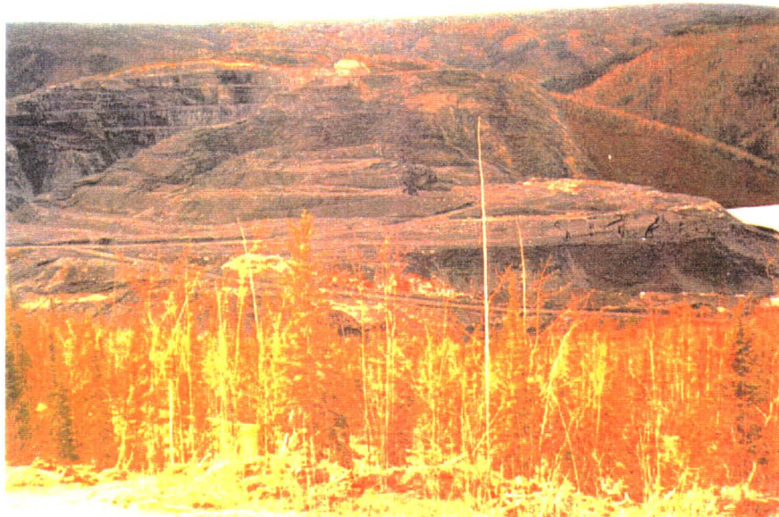
Photo 1: Tension Cracks at West End of Waste Rock Dump (1976)
