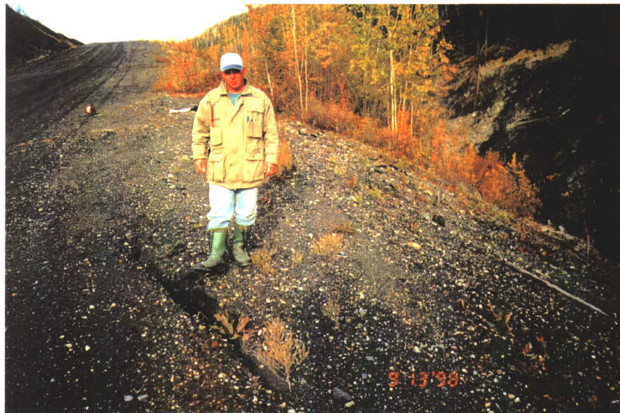
UMA Photo 7-14: Tension Crack Along Access Road (1998)
