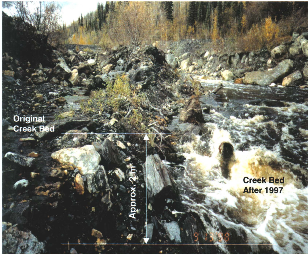
UMA Photo 8-13 Channel Down-cutting Immediately Downstream of Hudgeon Lake Outlet
