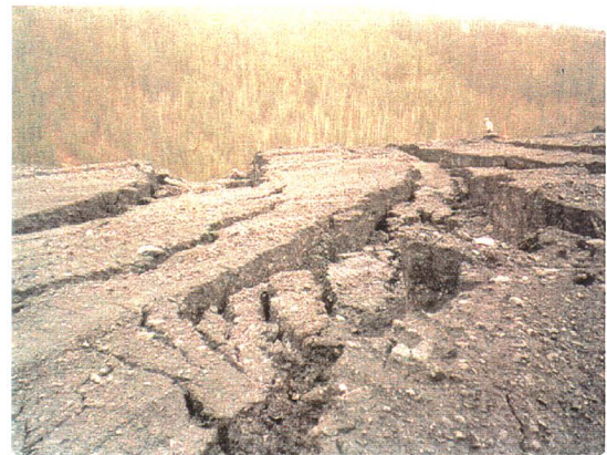
Cracks Near Crest (Mon #7 on Right)
