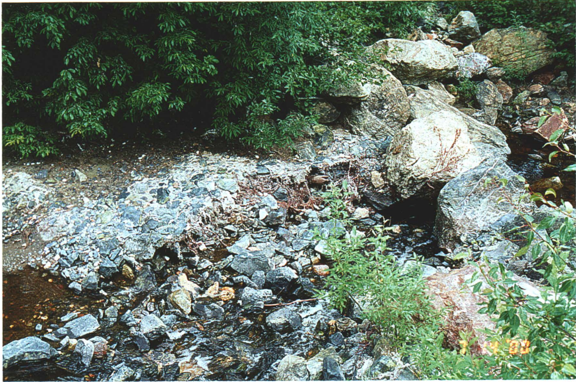
Photo 11: View of the Wolverine Creek lowermost rock weir, currently dislodged. Note the channel erosion.
