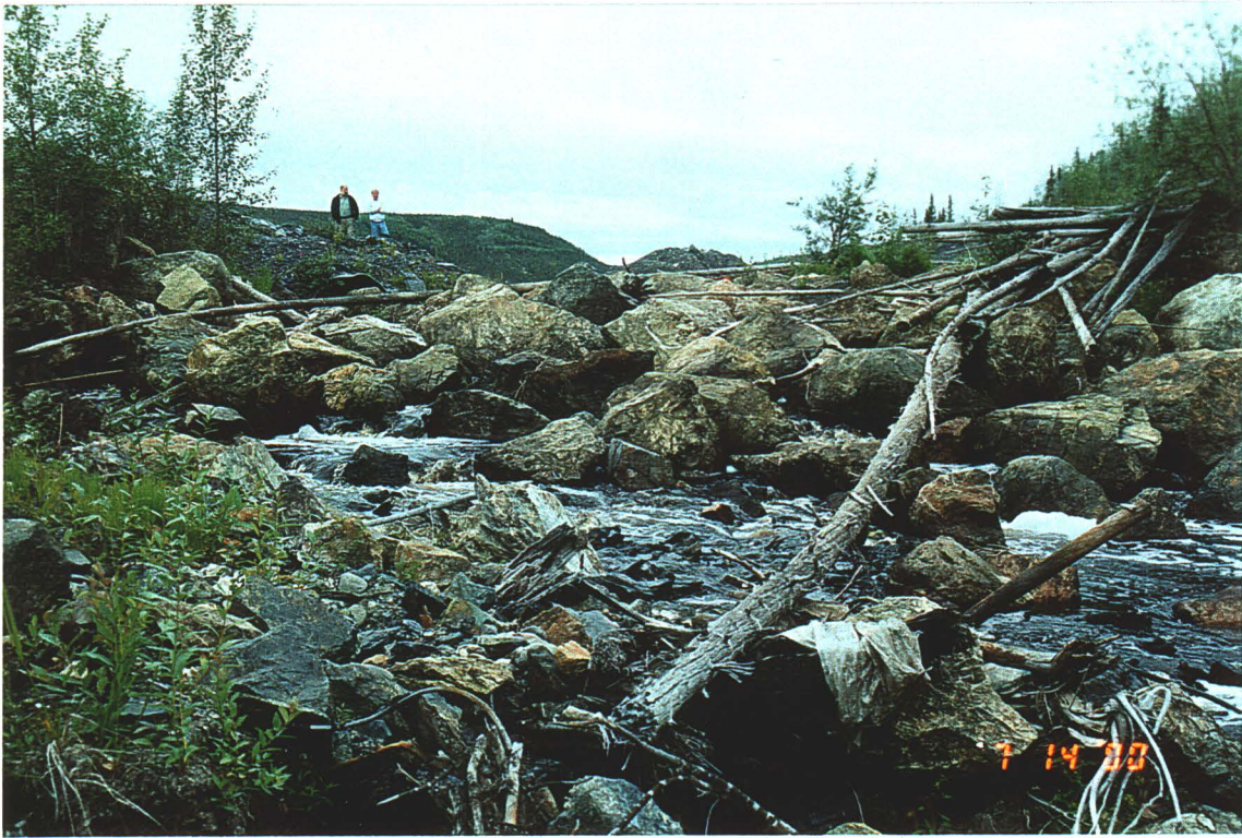
Photo 1: Looking upstream at the rip-rap segment of the Hudgeon Lake outlet. The left side appears to sag relative to the right side.
