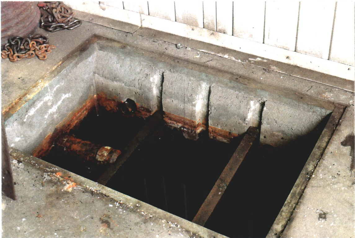
Photograph 6.10: Existing oil/water separator which receives floor drainage from the southern end of the maintenance building including the welding shop
