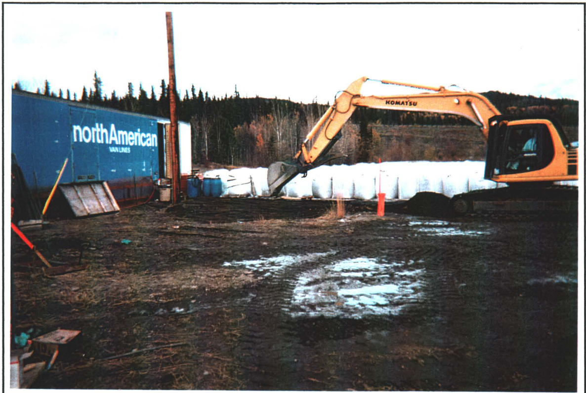
PHOTO 5: Excavator cleaning up area in front of Decontamination Van. Orange painted vertical pipe is location of piezometer.
