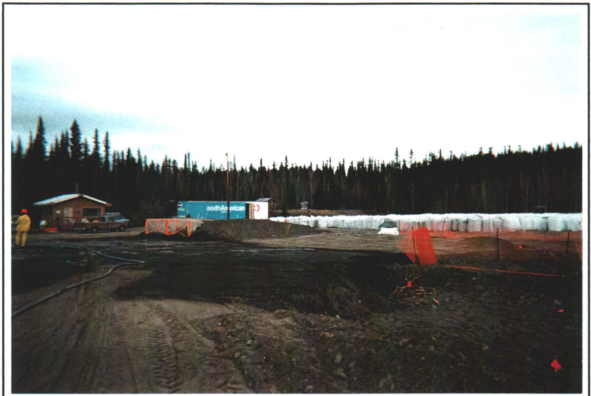
PHOTO 9: Backfilled and compacted area in northwest corner of excavation. Temporary ramp that is to be used to load trucks is visible at left.
