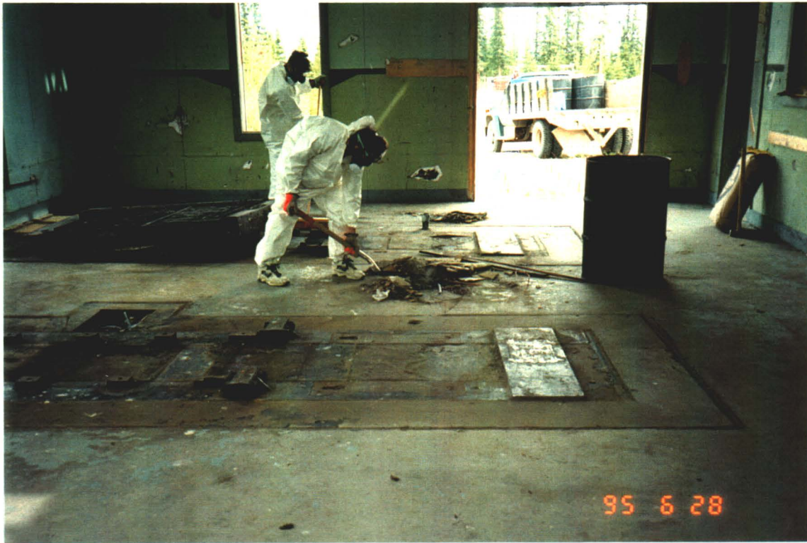
Photograph IV-1: Scattered debris from powerhouse floor containment in barrels.
