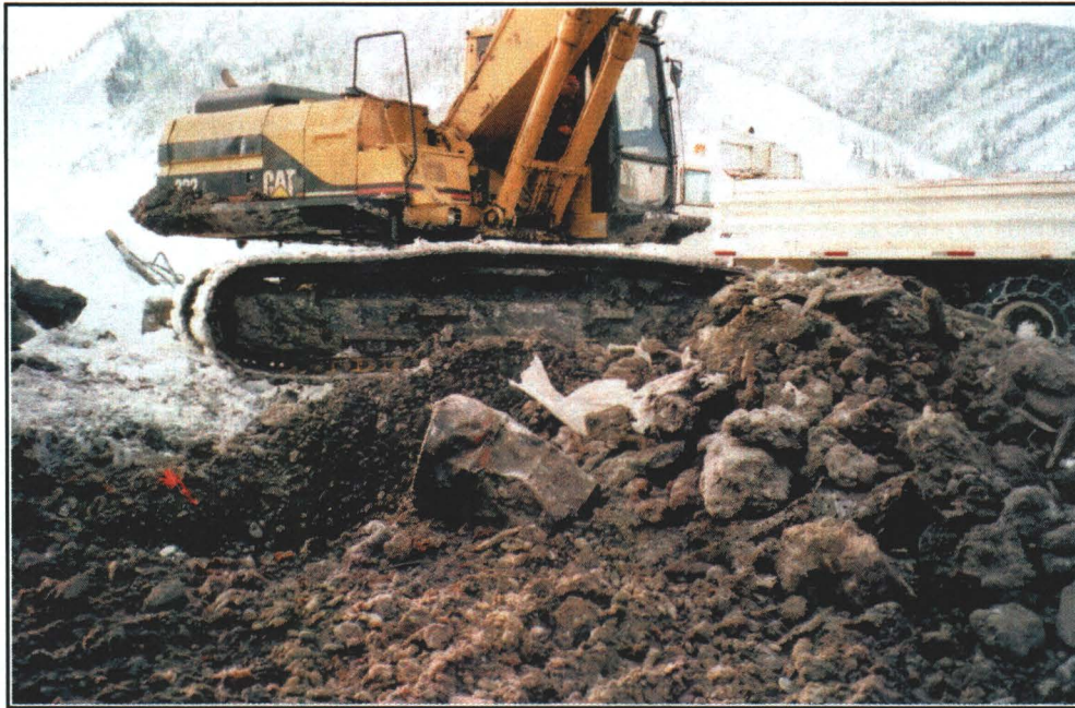
Photograph 2.9: Barrel and other debris excavated from the contaminated zone
