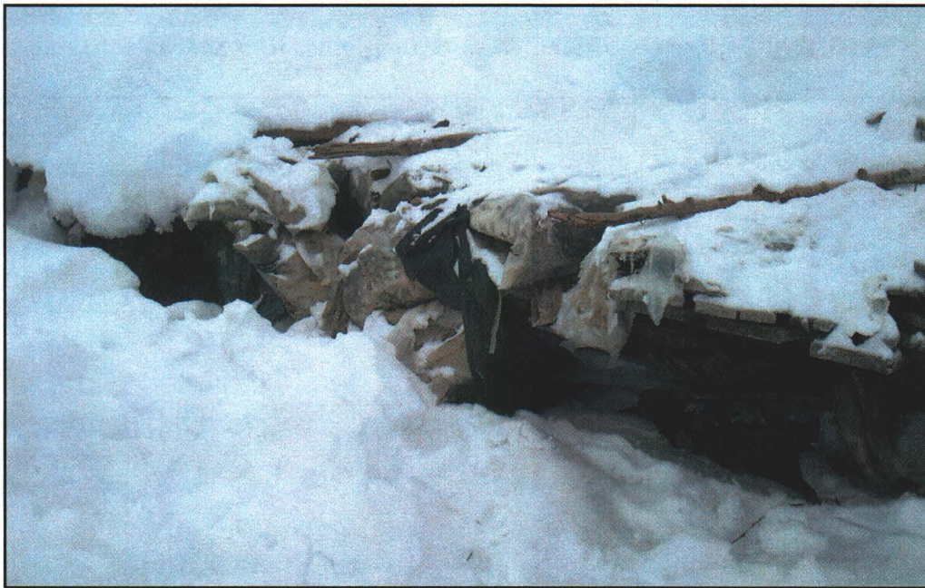
Photograph 2.13: Wood and other debris exposed along the cut bank prior to excavation
