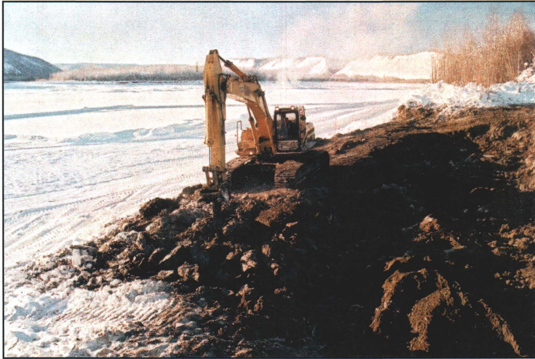
Photograph 2.6: Ripping the surface frost layer using a pick which was attached to the Cat 322 excavator
