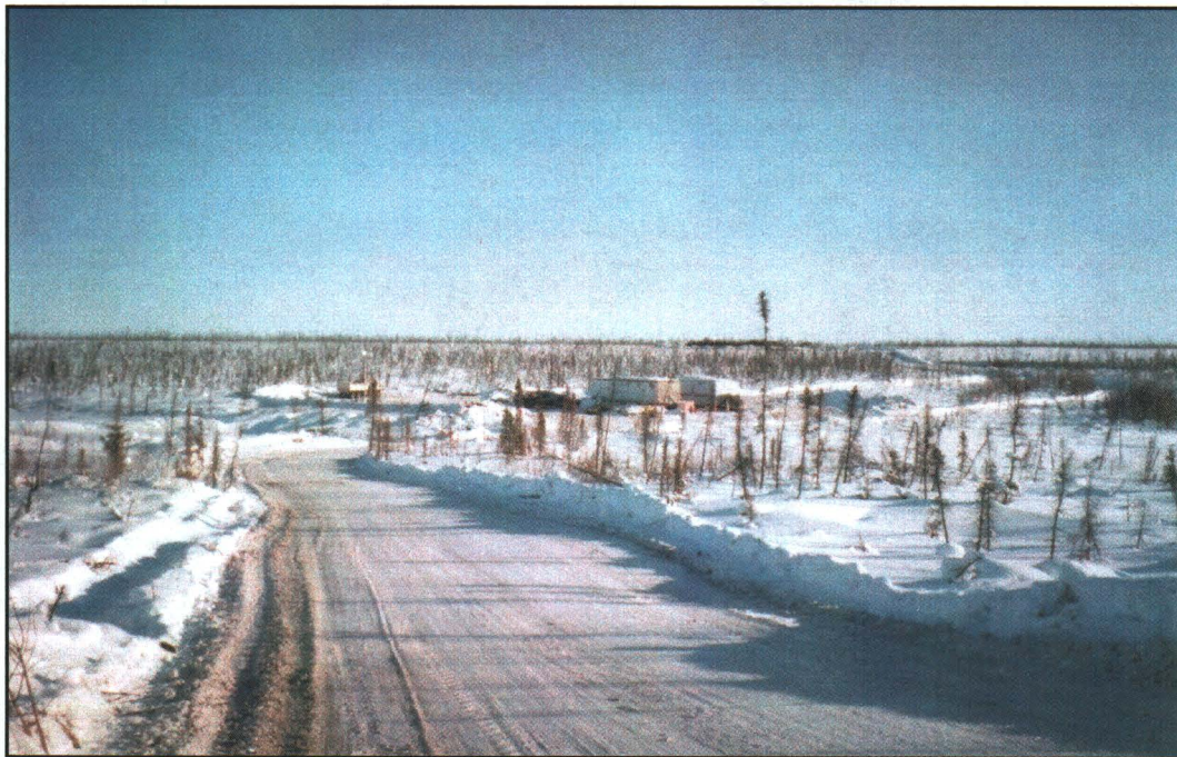
Photograph 2.2: View of the construction camp and part of the winter access road
