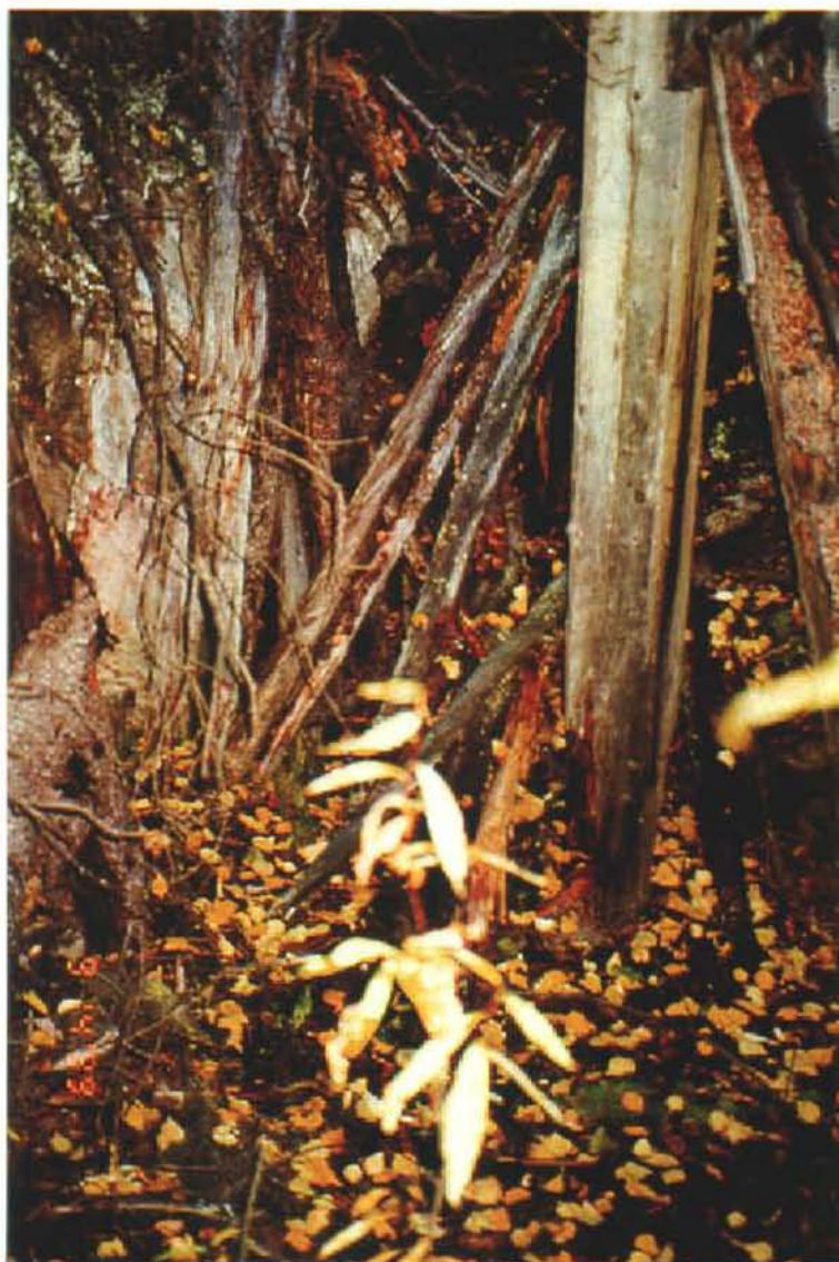
Photo 61-1: Timbers partially obscuring entrance to collapsed adit.
