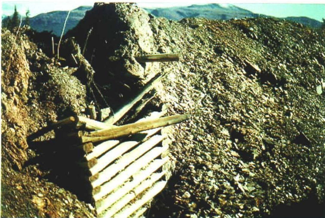
Photo 59-2. Collapsed shaft in center of trench.
