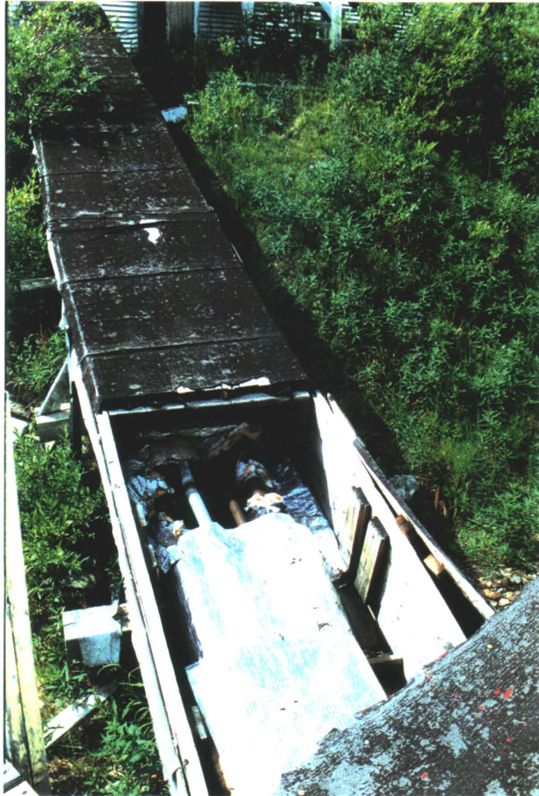
UTILIDOR WITH PIPING
