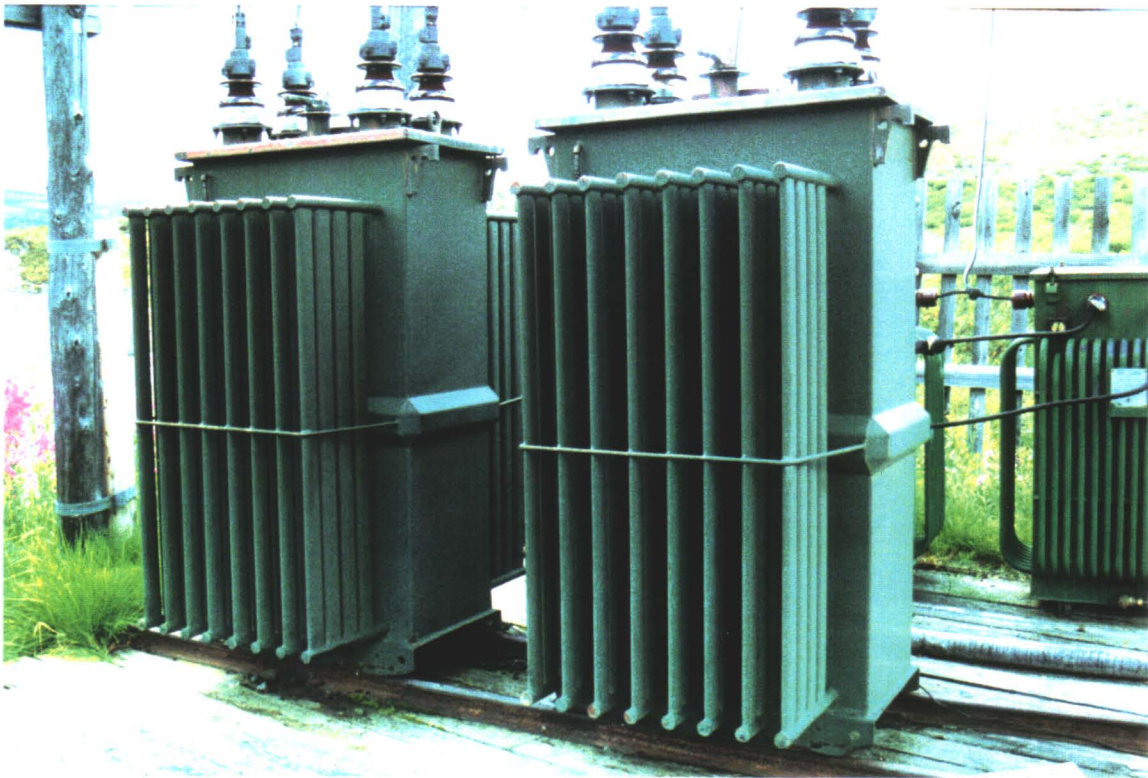
TRANSFORMERS AT LEVEL 700 SITE
