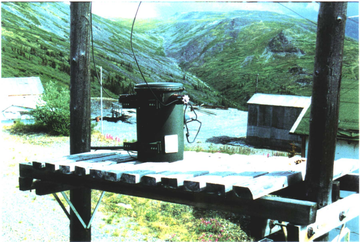
TRANSFORMER AT LEVEL 700 SITE
