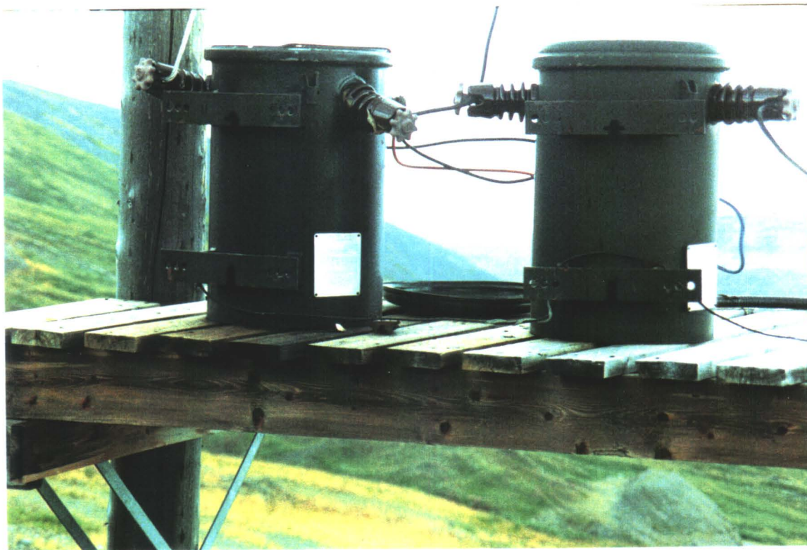
TRANSFORMERS AT LEVEL 200
