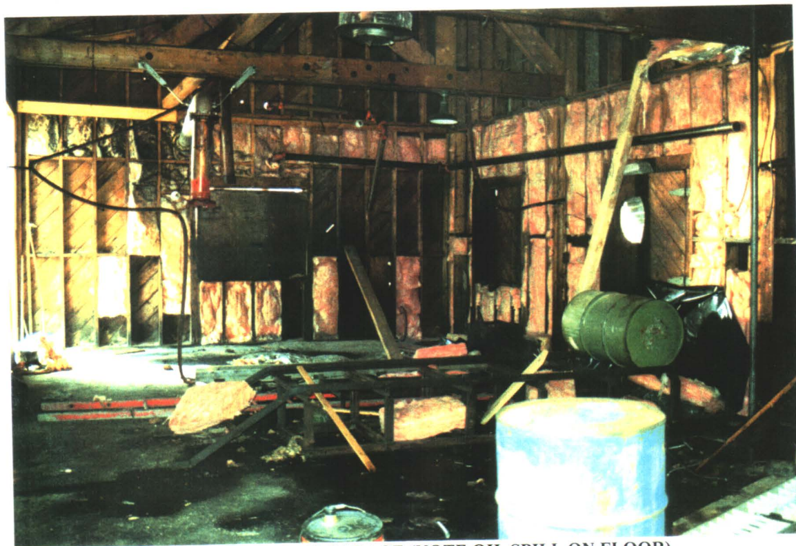
INTERIOR OF 4 BAY GARAGE (NOTE OIL SPILL ON FLOOR)
