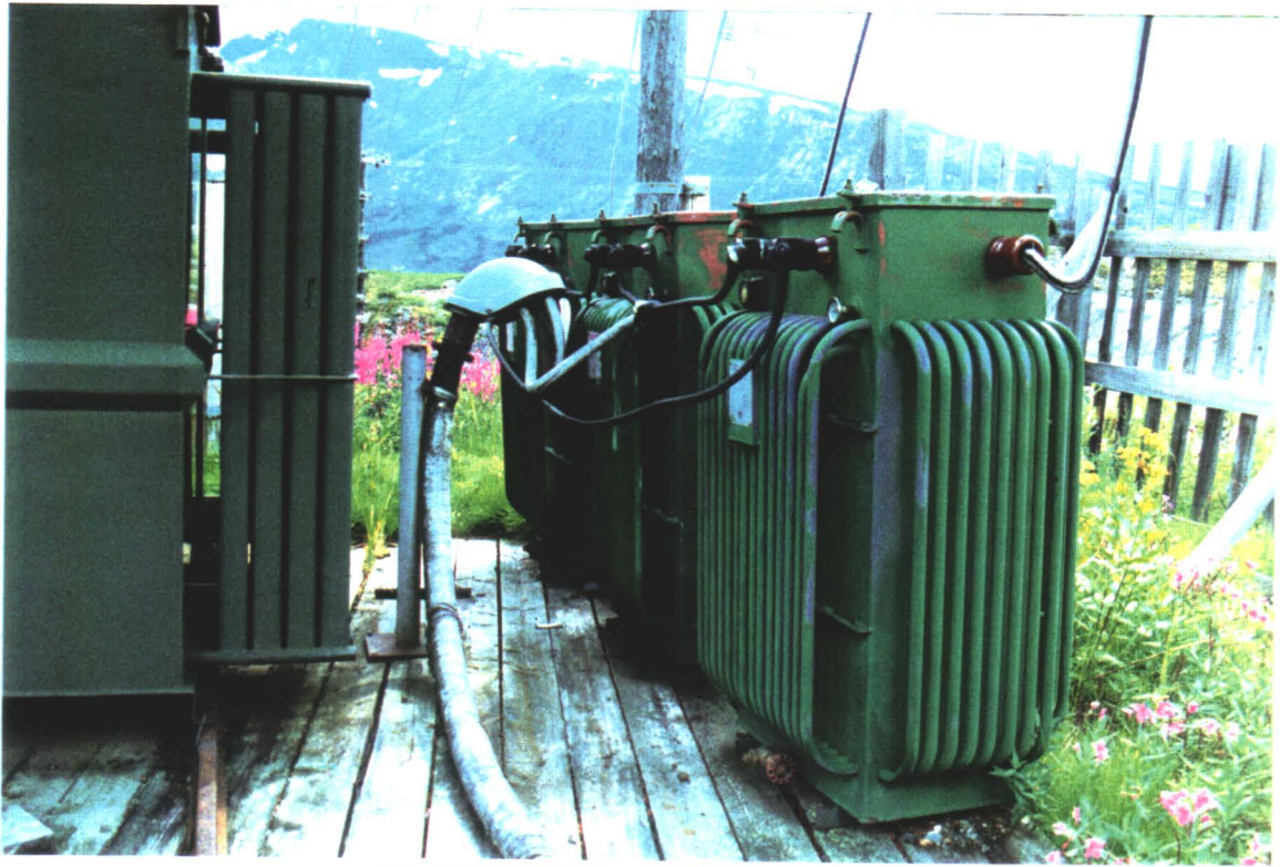
TRANSFORMERS AT LEVEL 700 SITE
