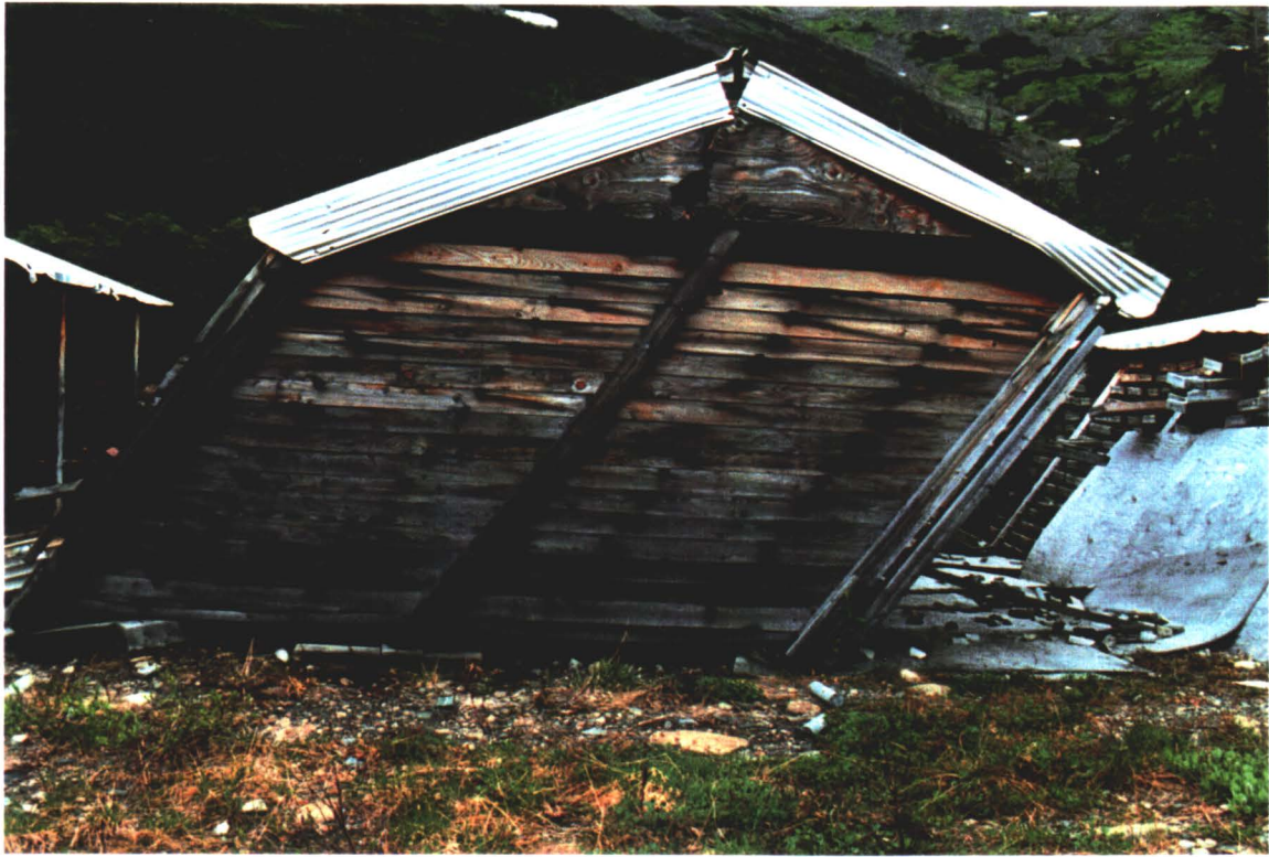
13. COLLAPSING CORE STORAGE SHED
