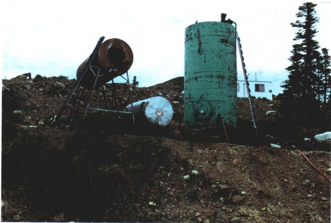
10. 2270, 4540, & 22700 LITRE FUEL STORAGE TANKS AT MAINTENANCE AREA
