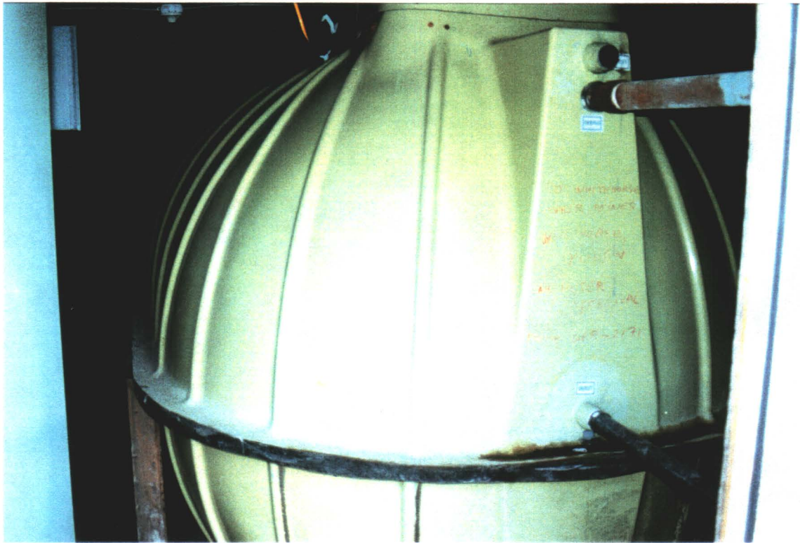
WATER STORAGE TANK
