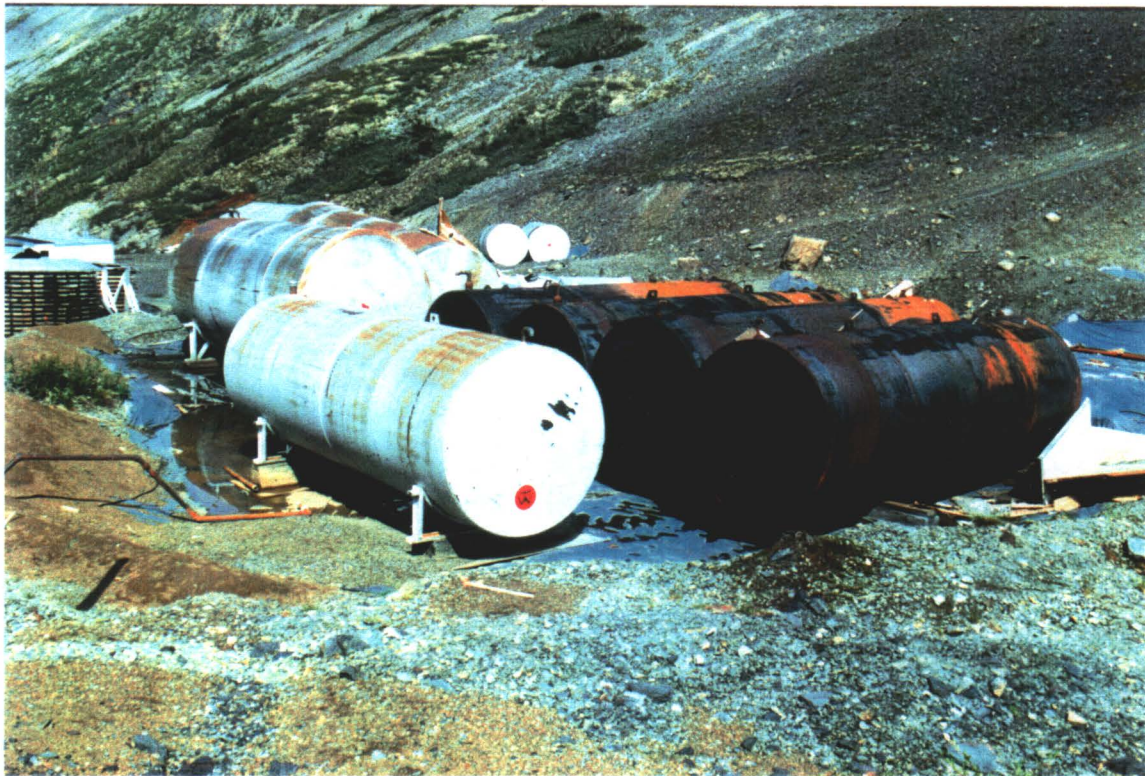
FUEL STORAGE TANKS
