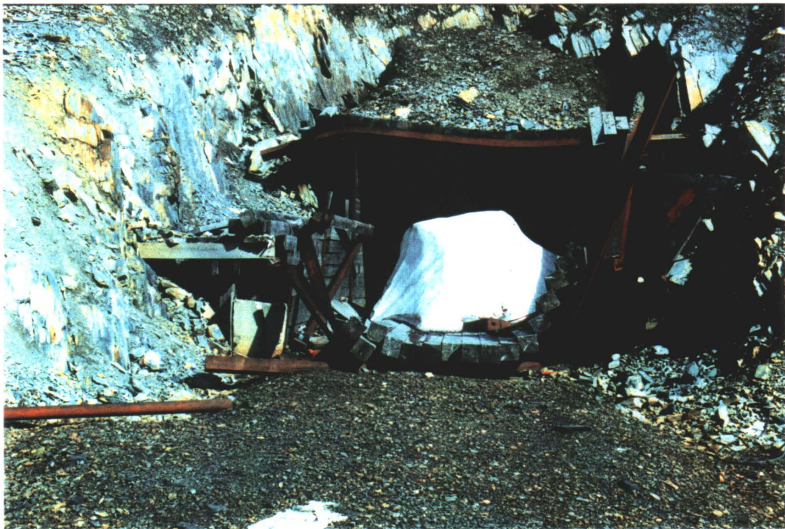
MAIN COLLAPSING ADIT WITH SNOW AT ENTRANCE
