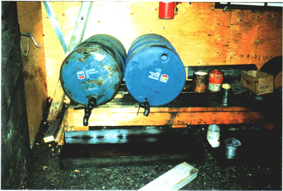
OPEN OIL BARRELS CONTAINING HYDRAULIC OIL INSIDE GENERATOR BUILDING
