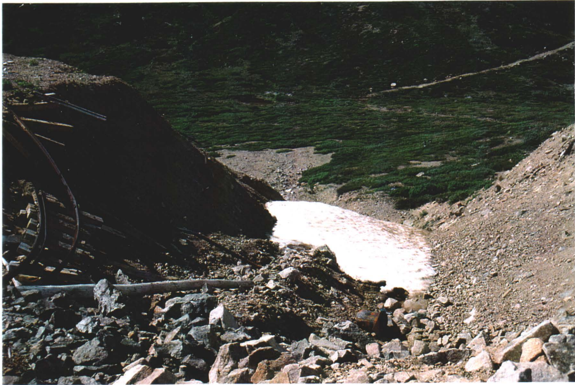
Photo # 15 - Twisted Track, Debris
