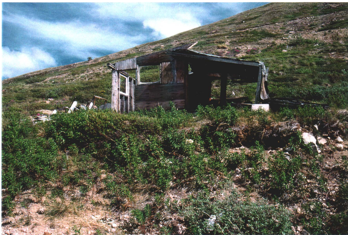
Photo # 2 - Collapsing Shack
