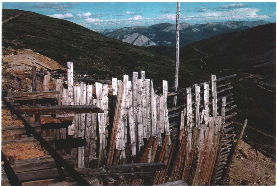
Photo # 12 - Dangerous Conditions - Loadout Facility
