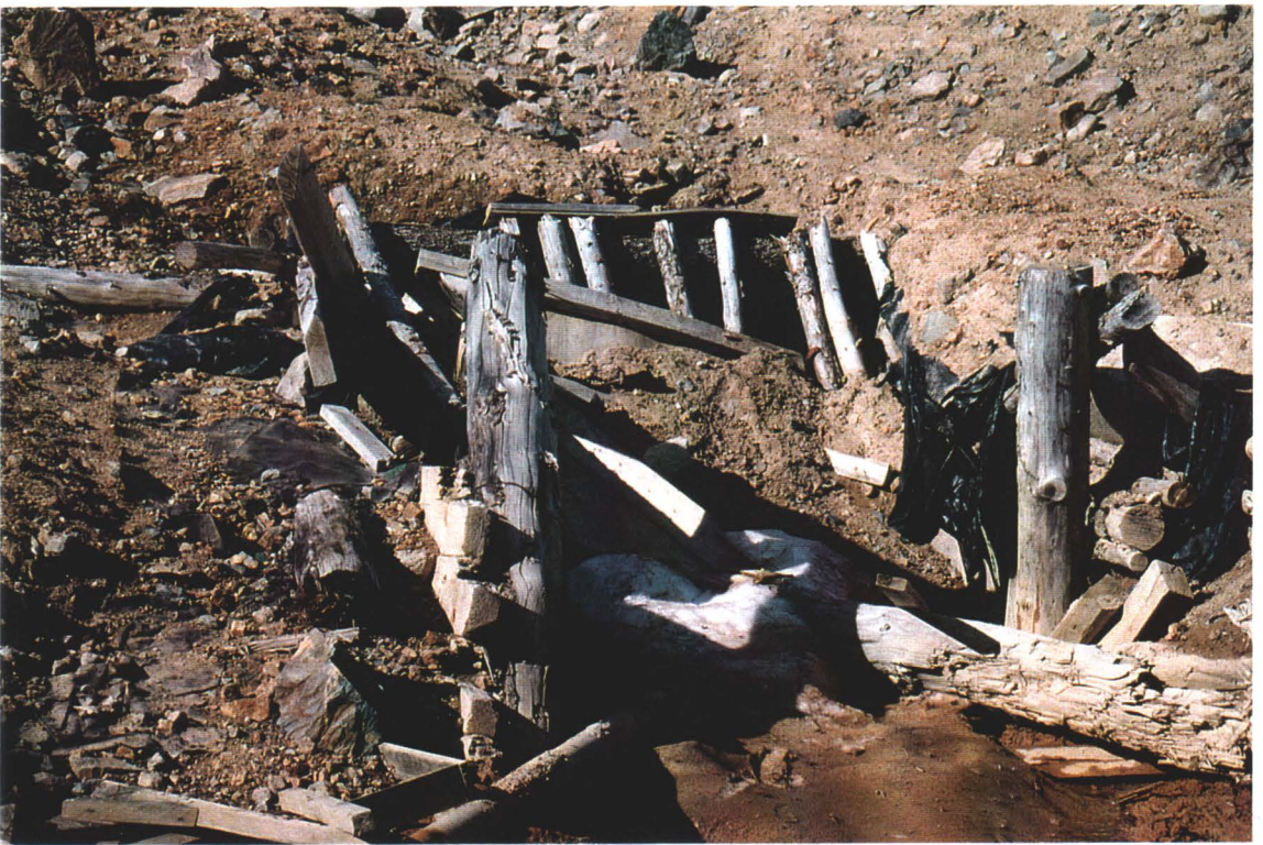
Photo # 30 - Lower Adit, Collapsed
