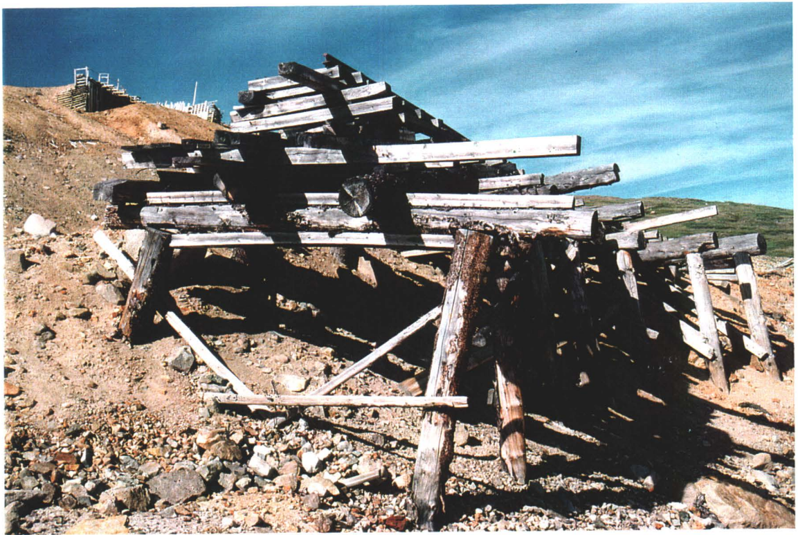
Photo # 26 - Loadout Facility - Deteriorating Condition
