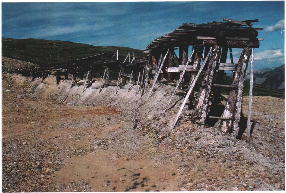
Photo # 25 - Loadout Facility - Deteriorating Condition
