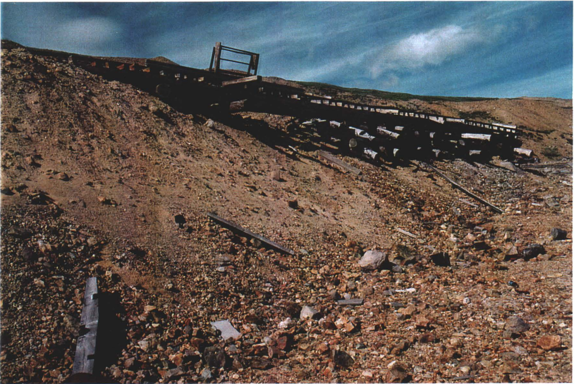
Photo # 14 - Dangerous Conditions - North Rails
