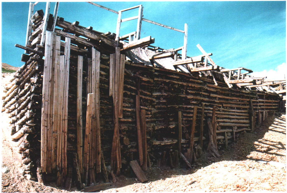
Photo # 11 - Deteriorating Structure - Detail
