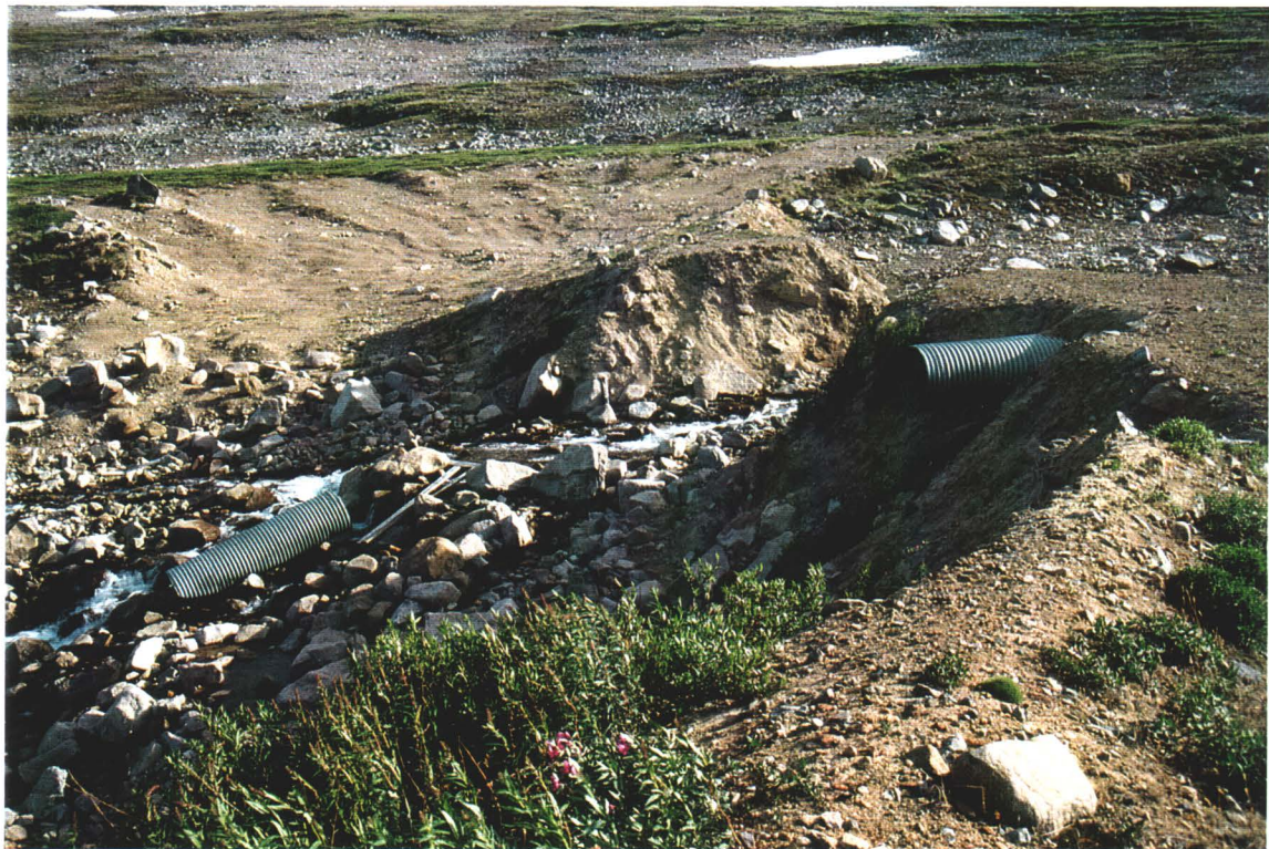
Photo # 39 - Culverts and Collapsed Dam
