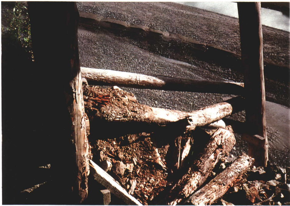
Photo 7. Timbers supporting the adit are in poor condition.
