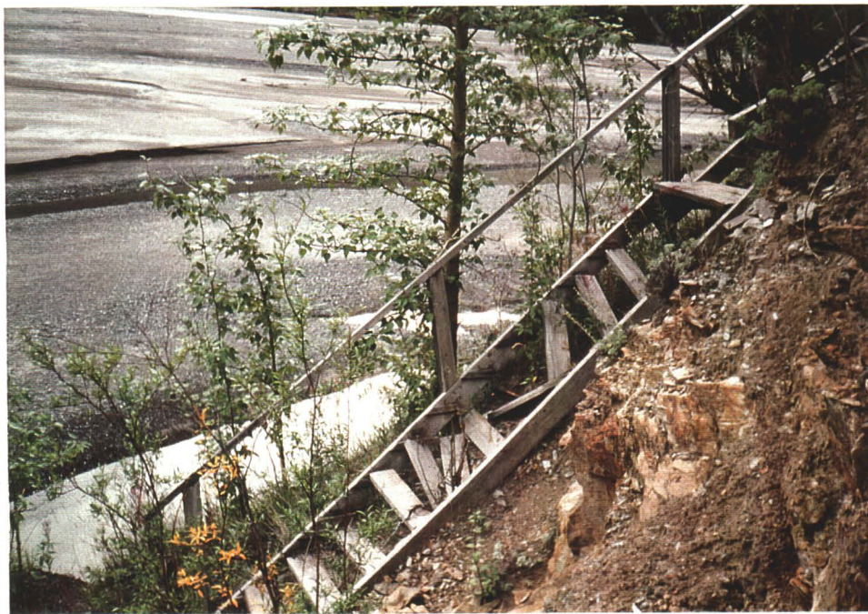
Photo 8. The staircase leading to the adit is in disrepair and is very unsafe.
