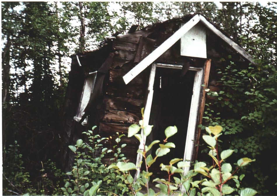
Photo 11. Damaged building at fringe of open area along side access road. In same general area as building debris shown in photo 10.
