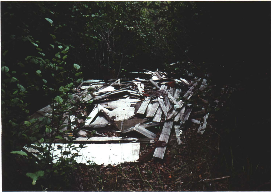
Photo 10. Demolished building in the wooden area on bank above the adit area.
