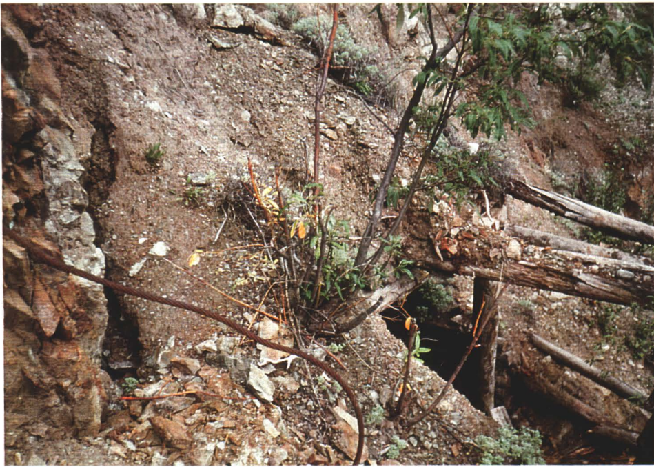
Photo 5. Bank area above adit opening. Note loose shale material on bank.
