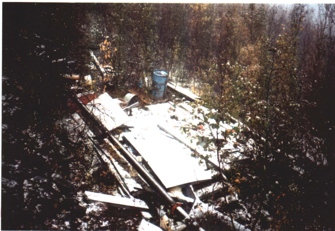
Photo 5: Foundation of compressor station/mine services shed, air pipe and assorted debris, looking northwest. September 19, 1996
