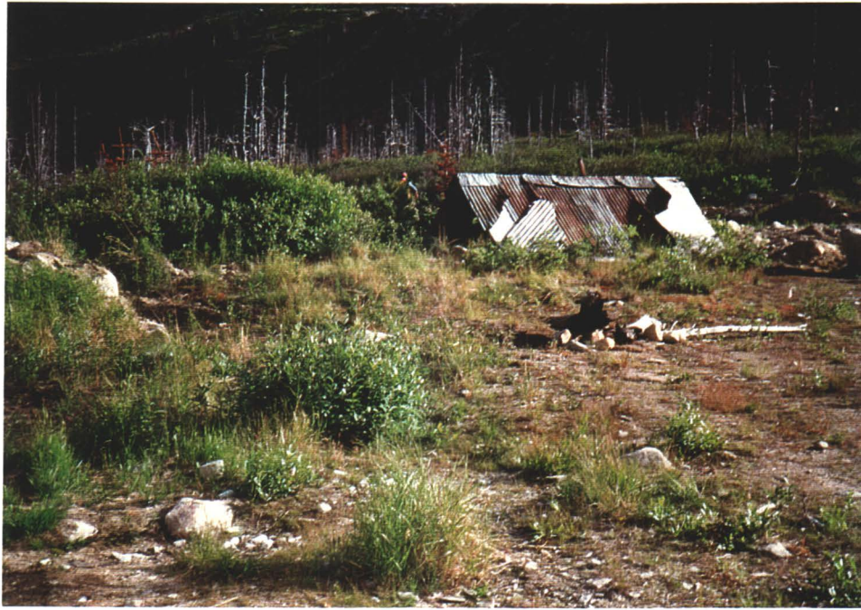
Photo 19. Wood frame metal clad A-frame former roof of log structure used for storage.
