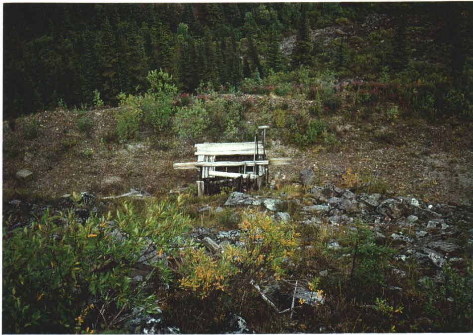
Photo 2. Top of shaft enclosure (looking north downslope) will not prevent entry to shaft.
