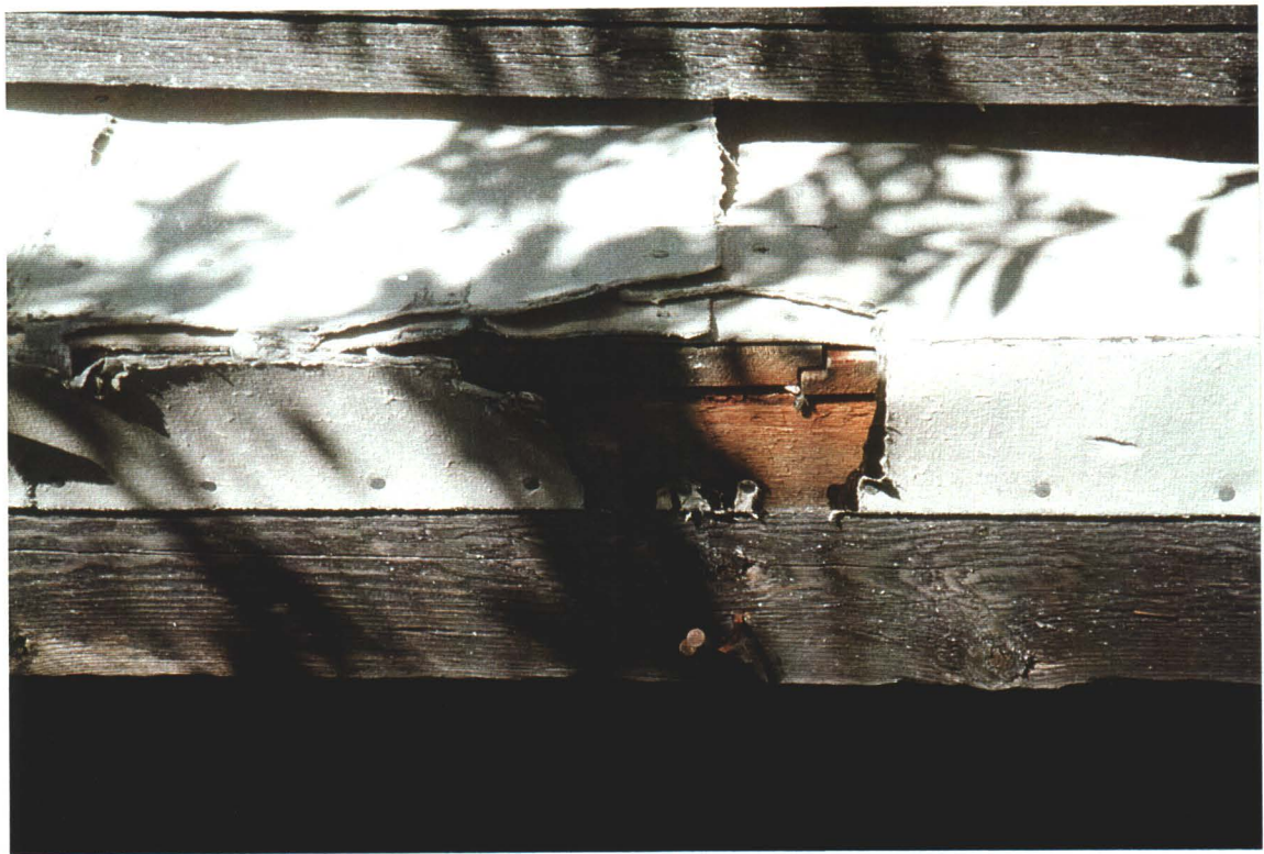
Photo 4. Asbestos-coated asphalt shingles on sides of core shed.
