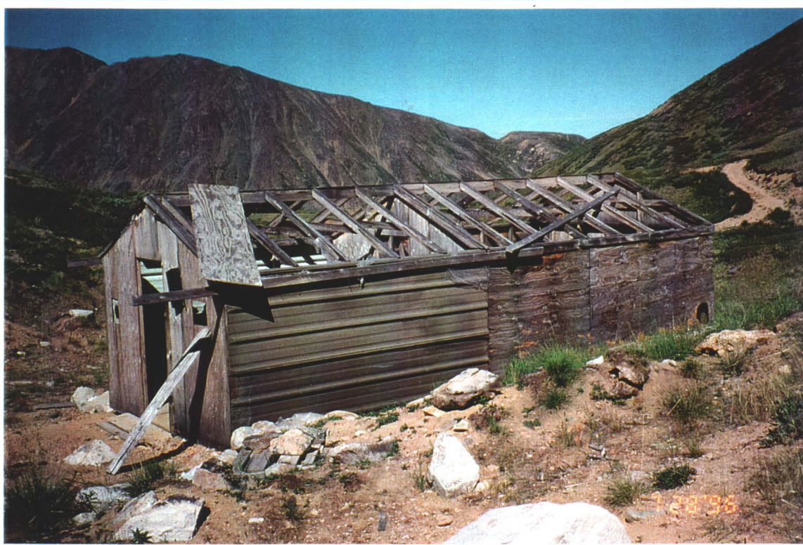
Photo # 1 - Deteriorating Shack on Site
