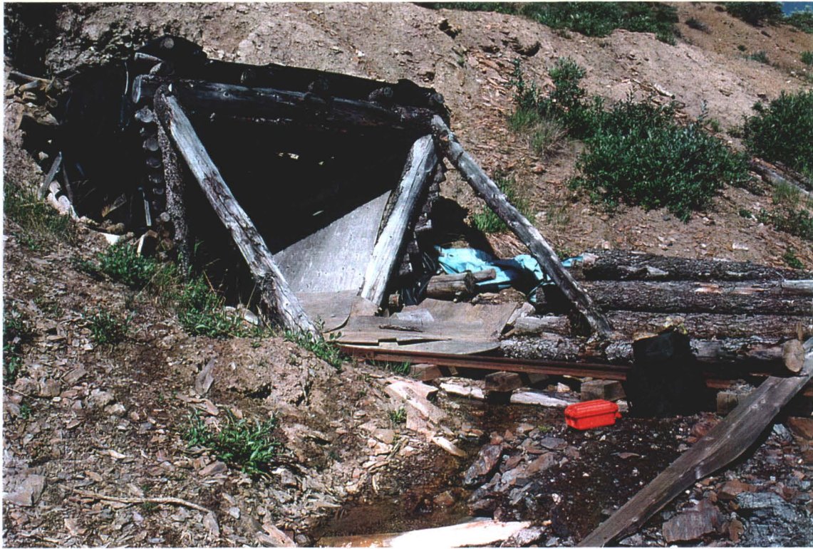
Photo# 9: Mine Water Seepage - Lower Site
