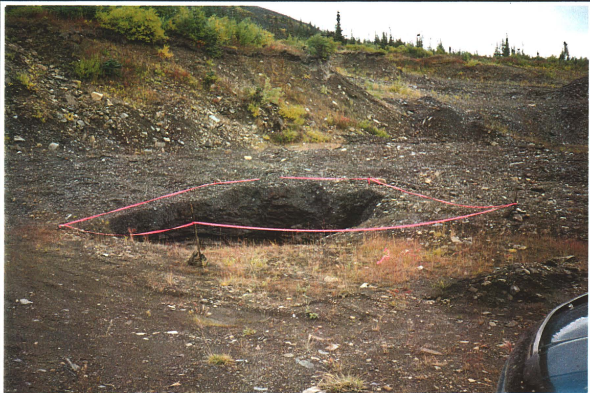
View of collapsed ground at centre of camp.
