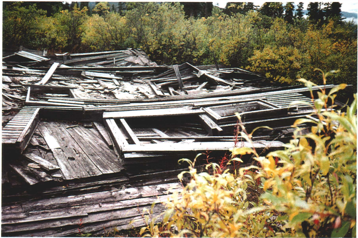
Collapsed building structure.
