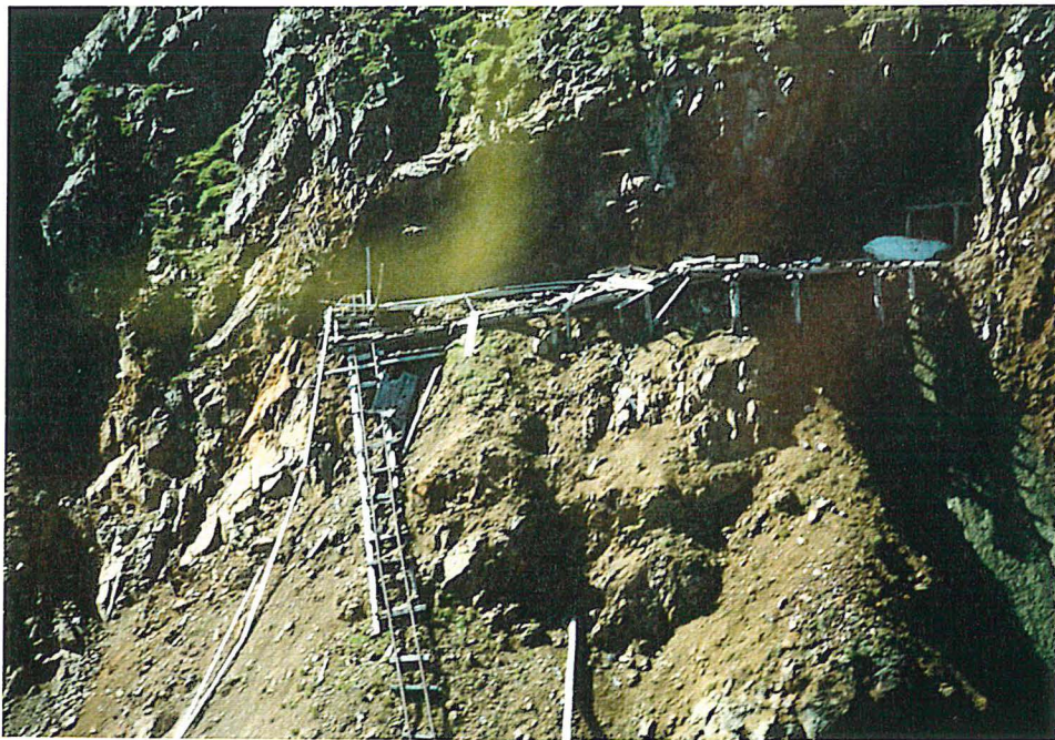
Photo 14. Track and trestle at Adit A2 (1707 m level). Note severity of slope, unstable surface and deteriorated condition of trestle and supports.
