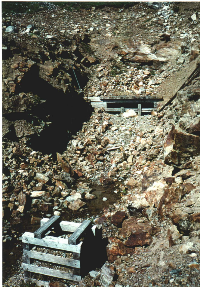
Photo 6. View from south of seepage from adit. Note collapsed conditions surrounding adit entrance.
