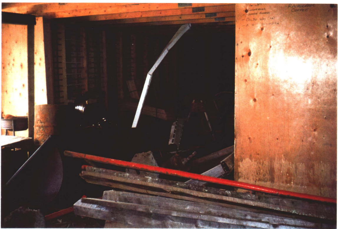
Photo 6. Wood and metal wastes, east side of core storage building.
