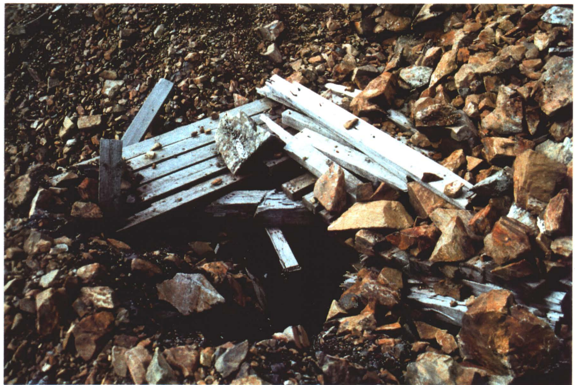
Photo 12. Adit near loading ramp, accessible through opening at lower centre of photo.
