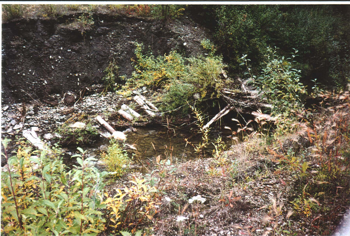
View of collapsed road and bridge at Lower Road.
