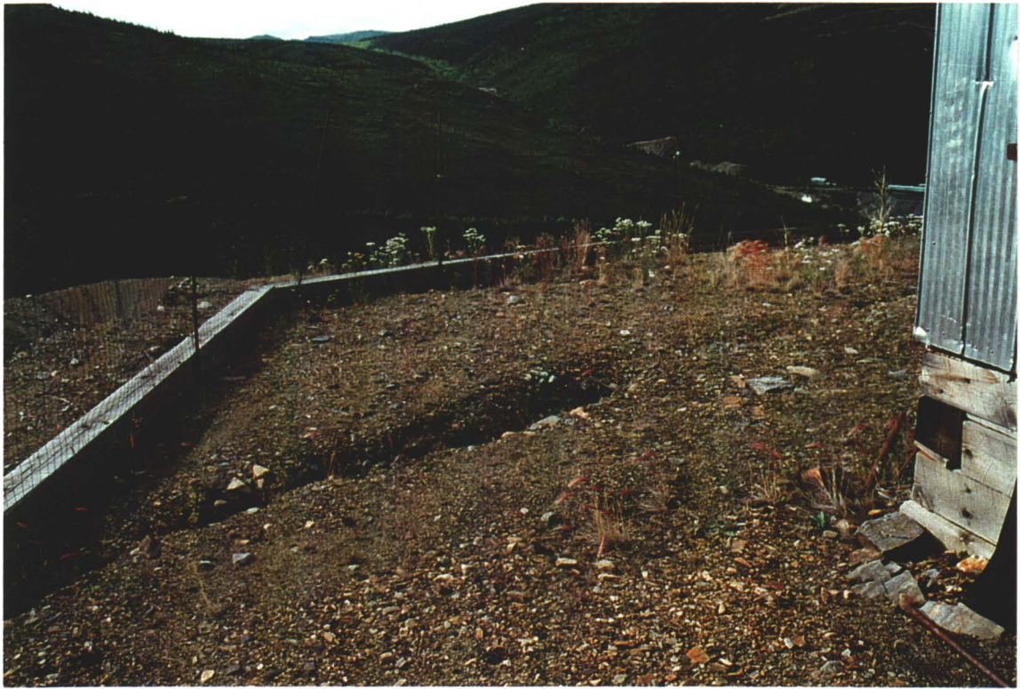
Photo 15. Slope failure crack within 3 metres of SE corner of garage.
