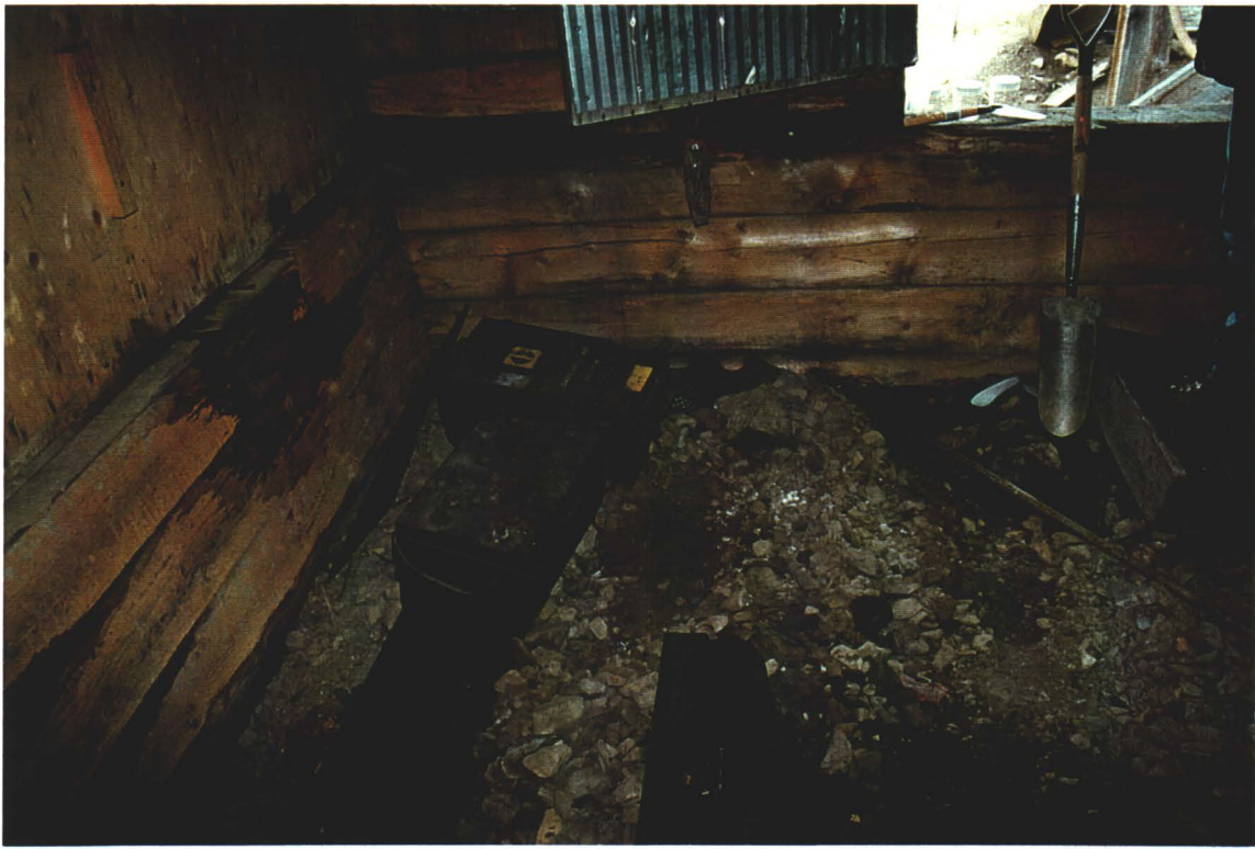
Photo 5. Interior of garage (looking toward doorway) with 2 Caterpillar tractor batteries and areas of soil staining visible.
