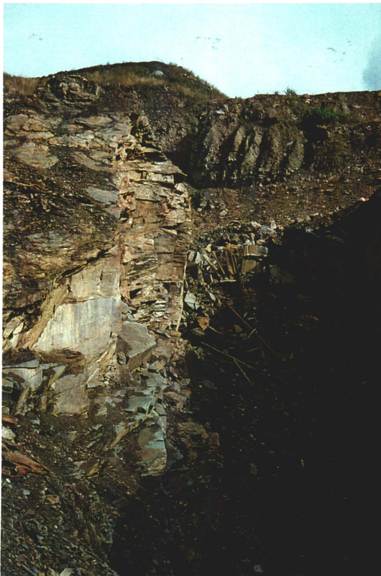
Photo 14. Collapsed adit entrance in lower trench (centre of photo). Note steep, unstable overburden above at top of trench.
