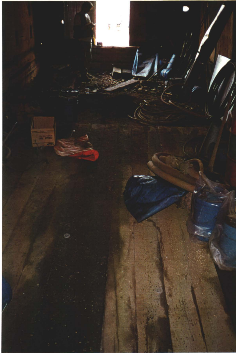
Photo 11. Interior of garage; note extensive hydrocarbon staining of timbered floorboards.
