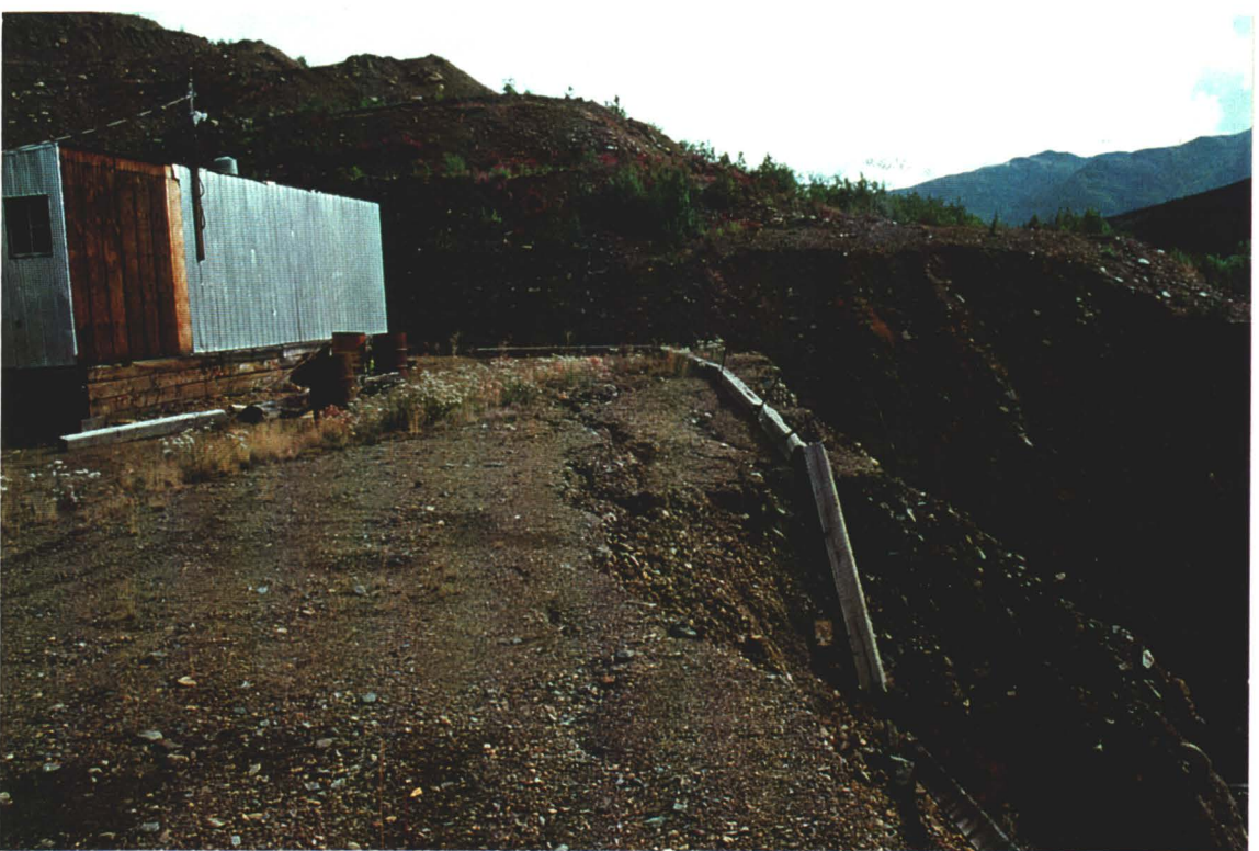
Photo 16. Slope failure cracks and "hanging fence" near garage, looking northeast.
