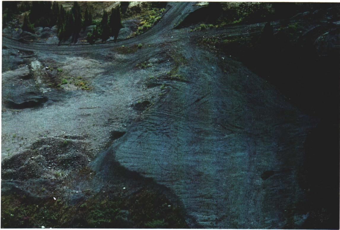
Photo 5. Waste rock pad constructed near mine access road at base of slope.
