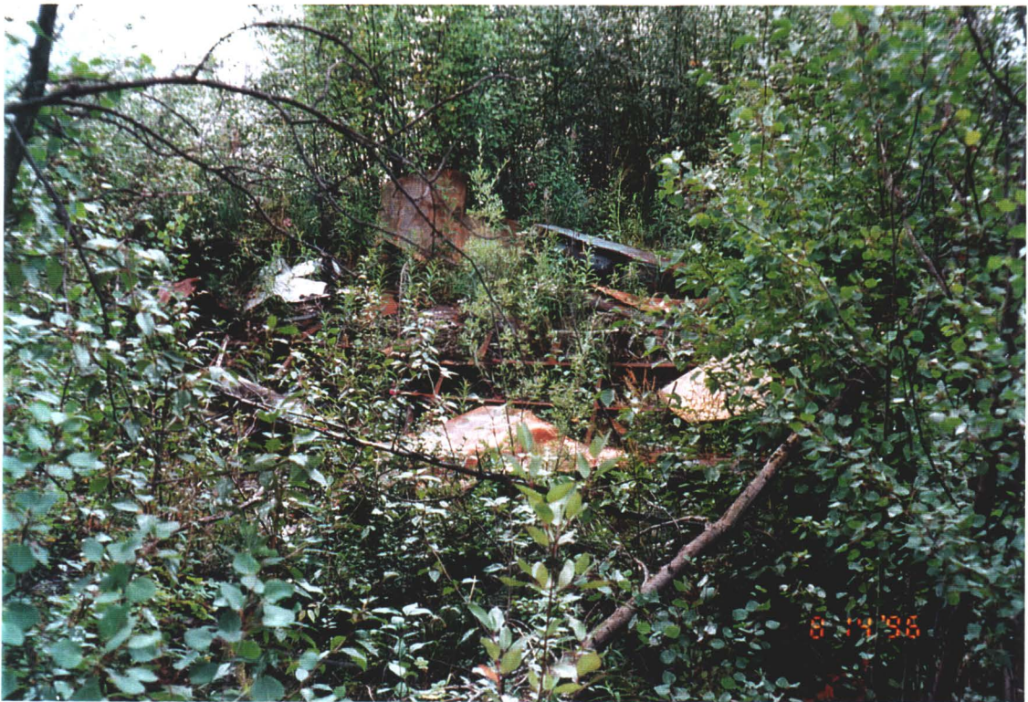
Photo # 8 - Remains of Collapsed Office Trailer near Metal Dumpsite
