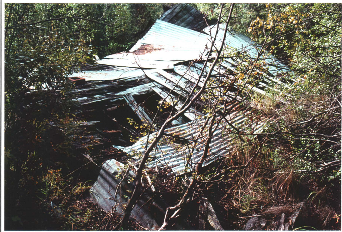
Photo # 8 - Maintenance Building (Collapsed)
