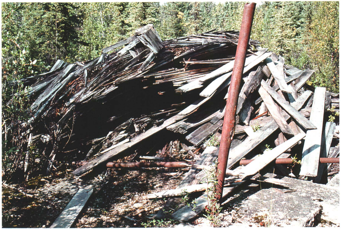
Photo # 20 - Collected Wood Debris west of Powerhouse
