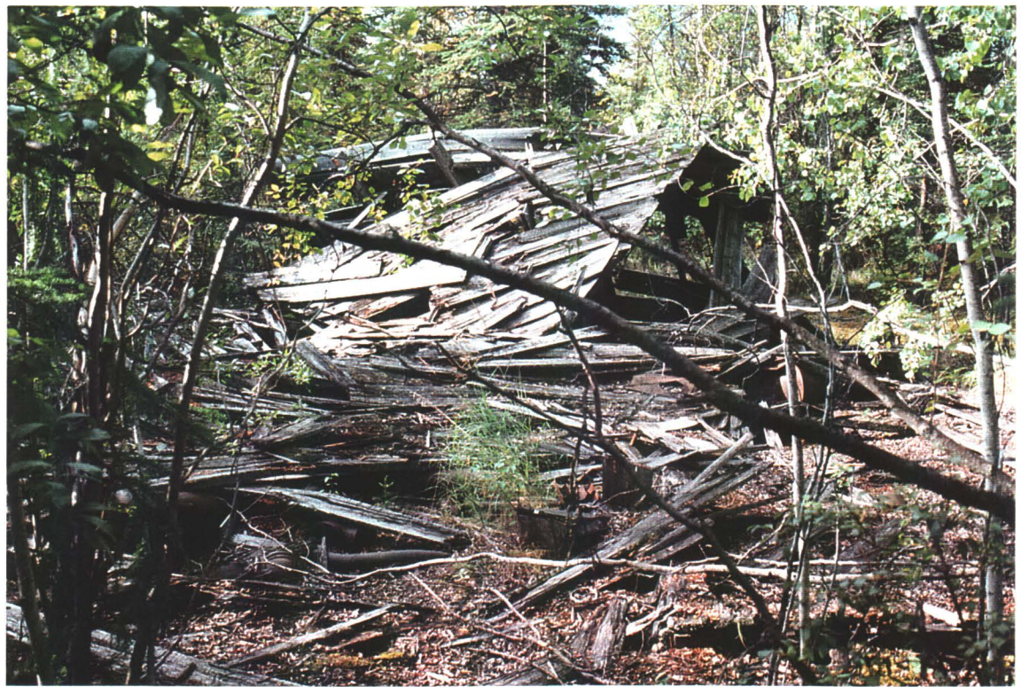
Photo # 13 - Warehouse Building (Collapsed)
